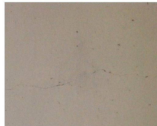
Hairline crack to 5 th Floor Slab
