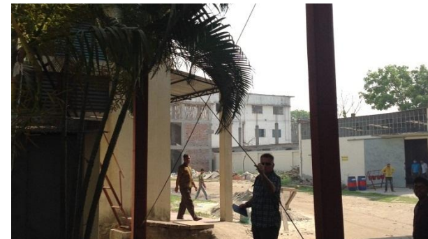
Loose Vertical Bracing to Entrance Canopy Frame
