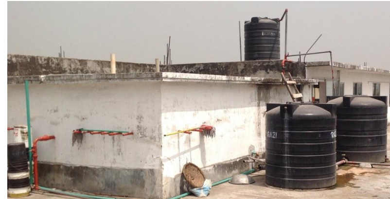
Water Tanks at Roof Levels
