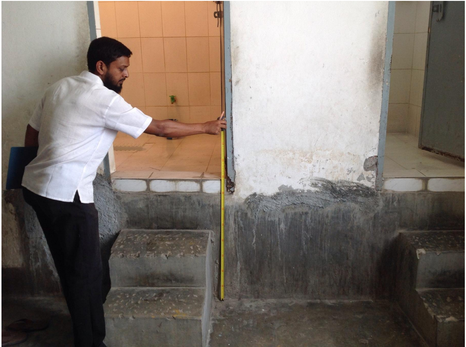
Possible 800mm Build-up (Average) in Toilet Area to South Staircore Half-Landing to all Floors
