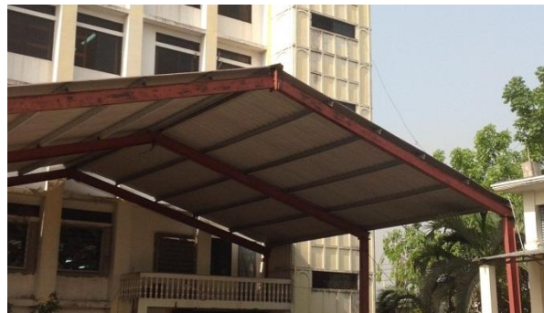
Lack of Horizontal Bracing to Entrance Canopy Roof
