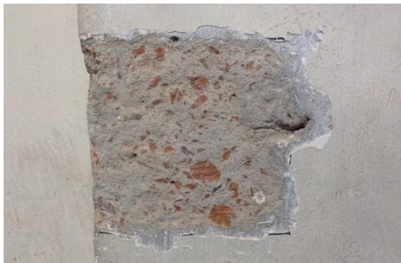
Tested Column - Arup
