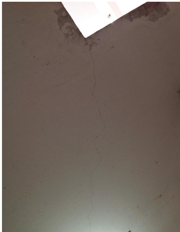
Hairline Cracking to Soffit of 6 th Floor Slab
