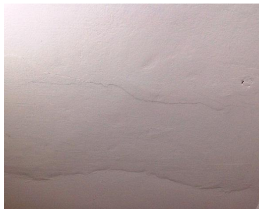
Hairline Crack to 3 rd Floor Slab
