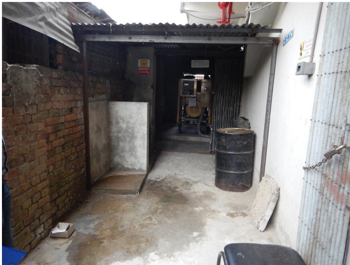
Water leak leading to structural damage
