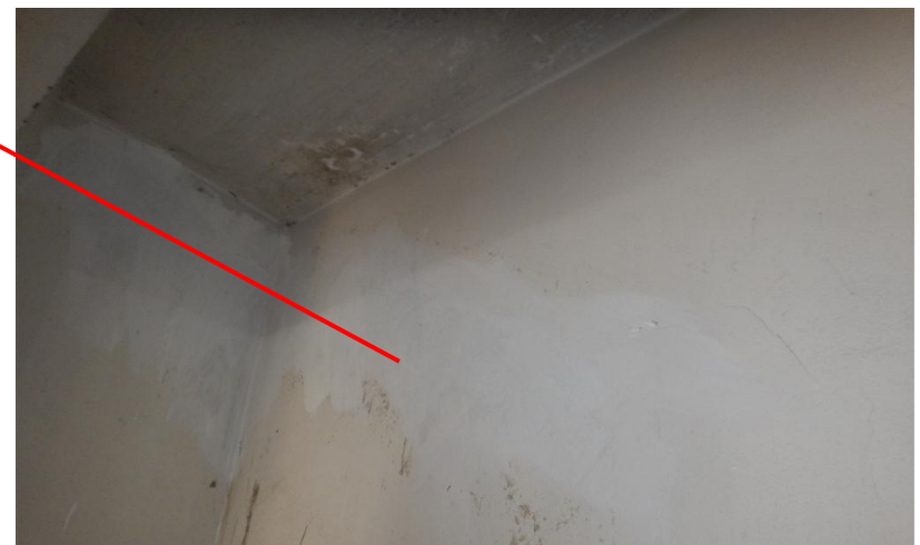
Horizontal and diagonal cracking observed in masonry wall directly below water tanks
