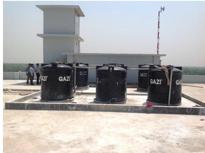
6 no. 2000 litre water tanks at roof level
