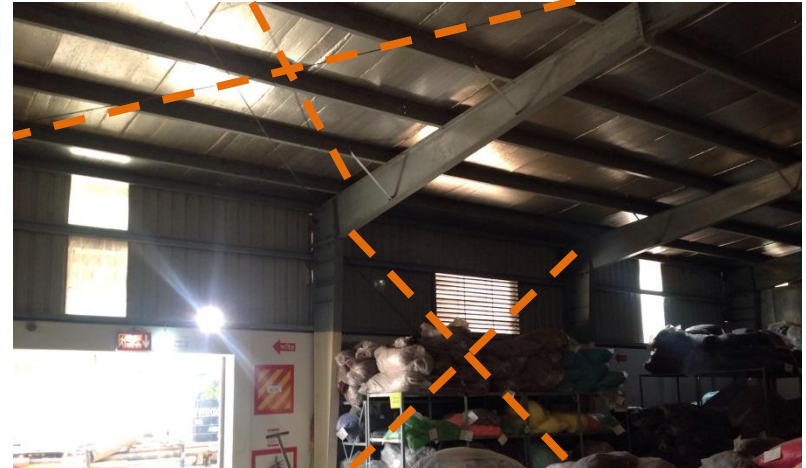
Godown Shed – discontinuity of vertical and roof bracing with no apparent eaves beam to transfer loads
