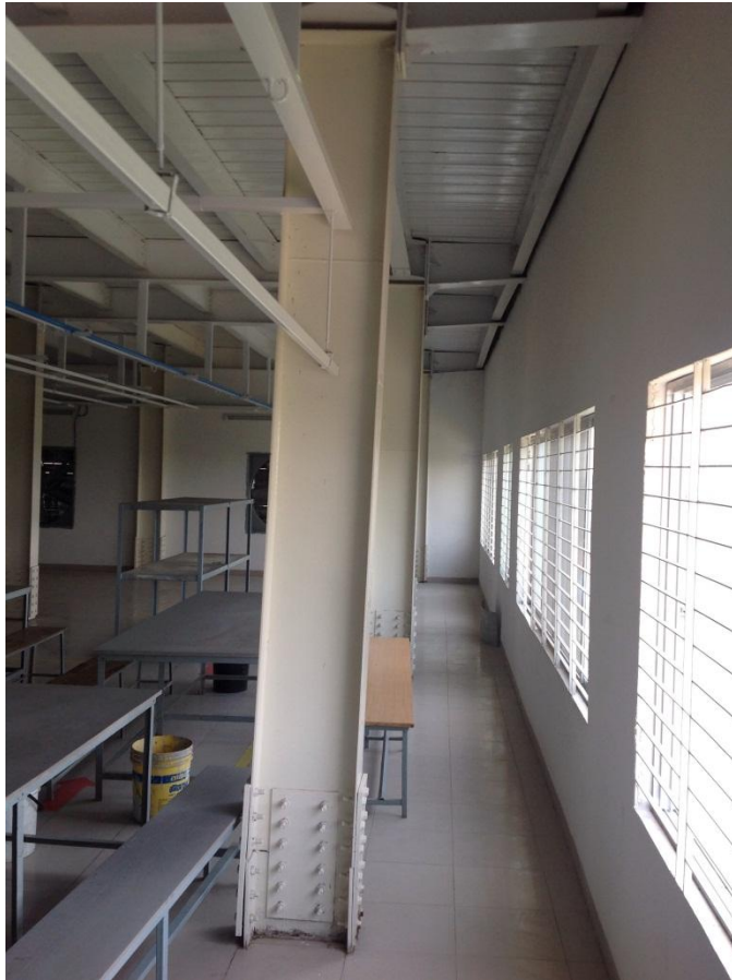
Columns out of plumb at 5 th floor
