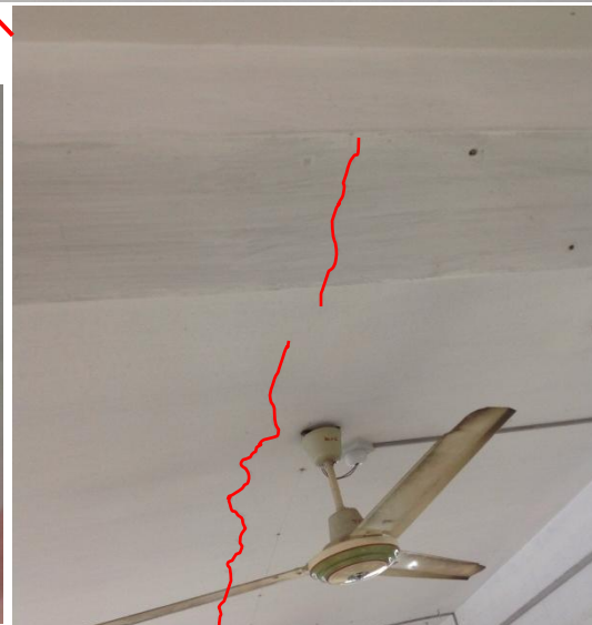
2 nd Floor crack in slab soffit
