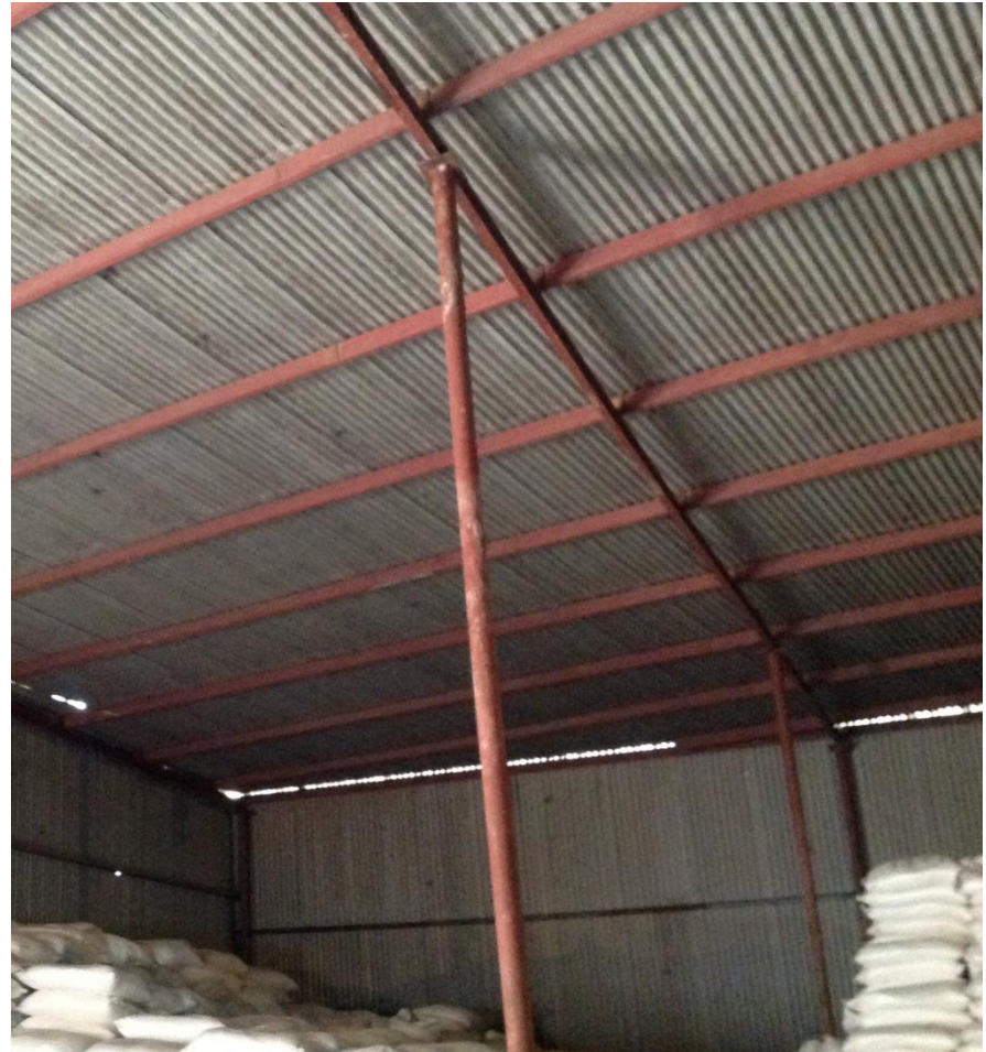
Columns at Risk of Corrosion
