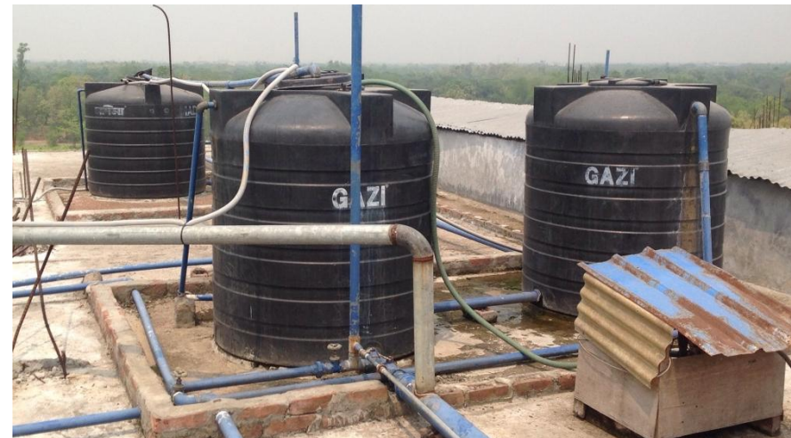
Water Tanks to Roof
