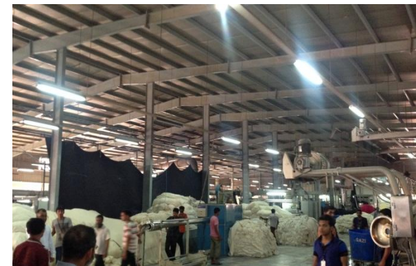
Bracing system missing from Dyeing Building
