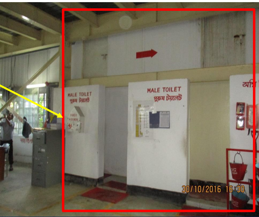
Missing vertical bracing at south side.
