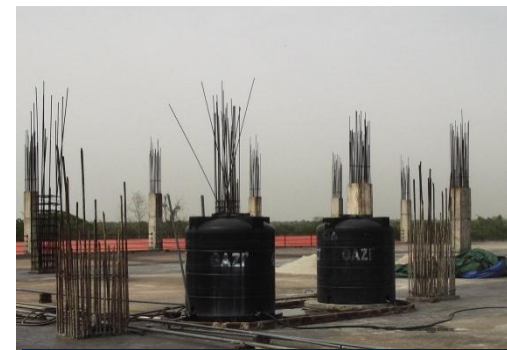
Water tanks loads
