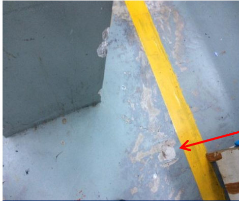
Cracks in 1 st floor slab
