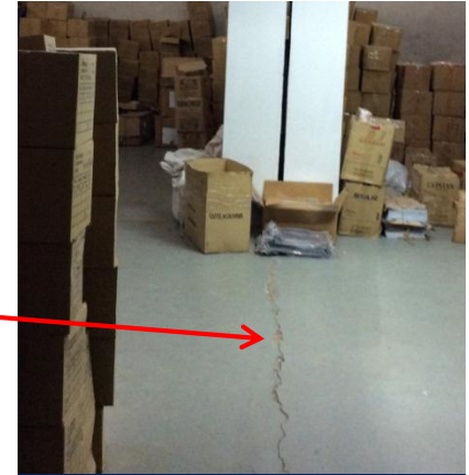
Cracks in Ground floor slab
