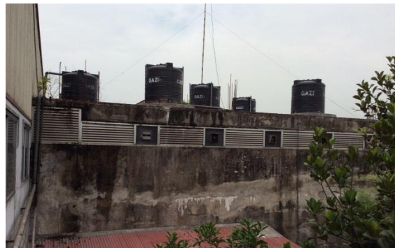
8 No. 2000 litre water tanks above the East extension
