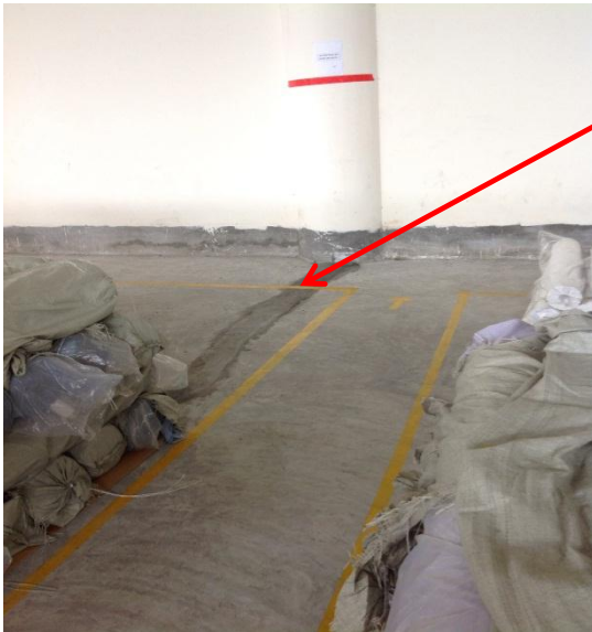
Extent of cracking
