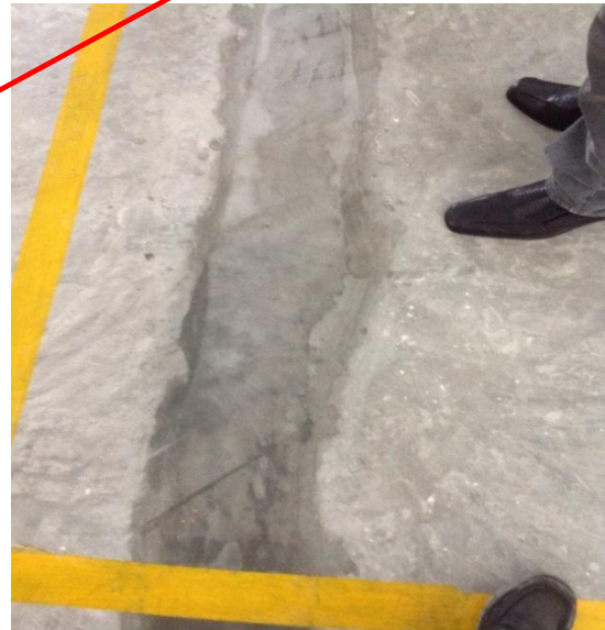
Crack over ground tie beams
