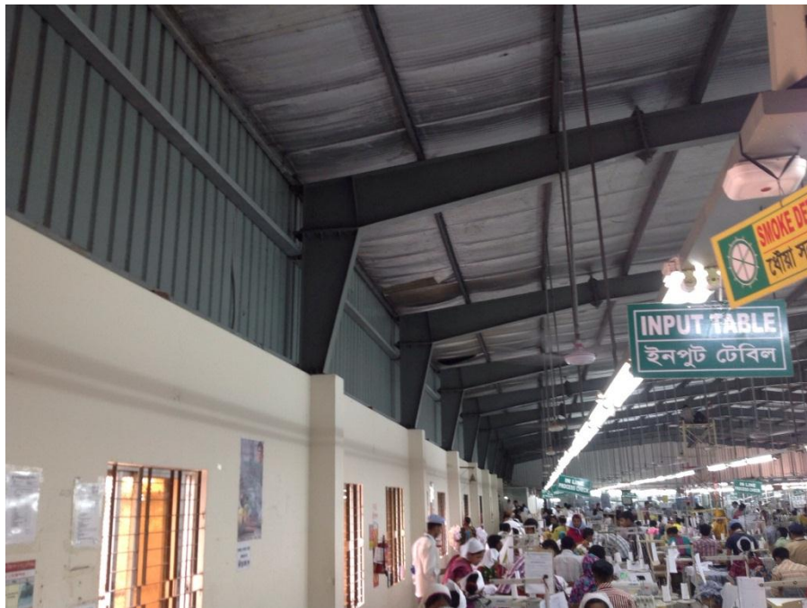
Eaves beams missing to Main Production Building
