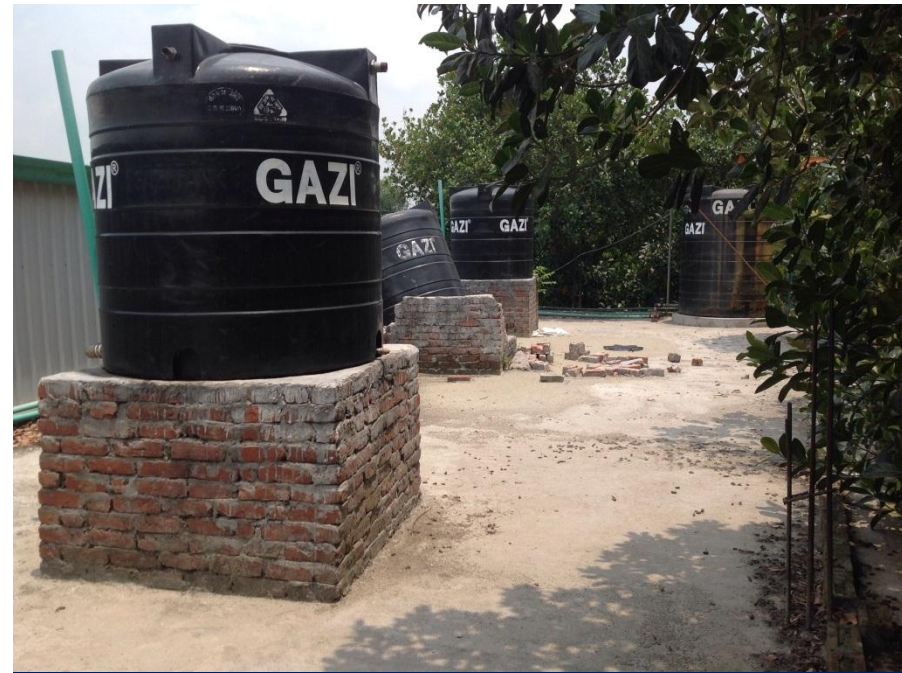
Water Tanks to Roof
