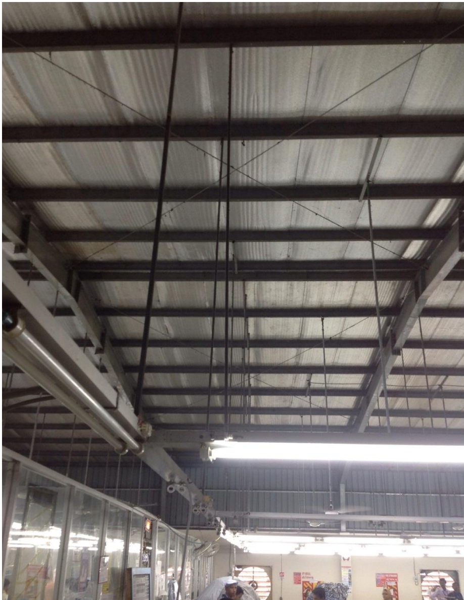
Vertical bracing system missing to Main Building
