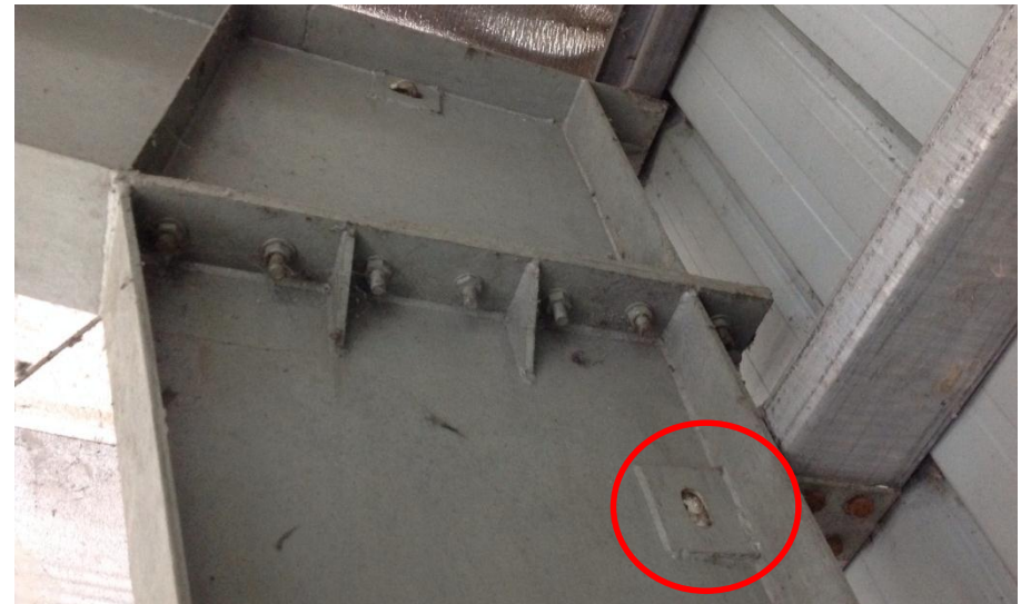
Bracing connection detail for horizontal bracing is provided to stanchion but not used. Eaves beam missing.
