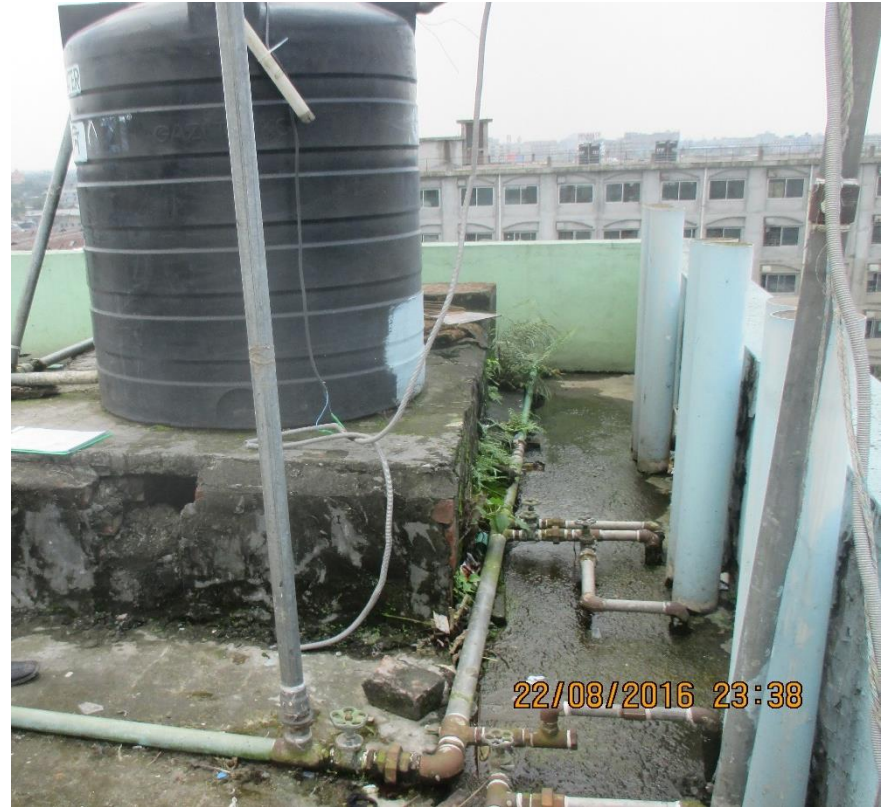
Sign of standing water was visible
