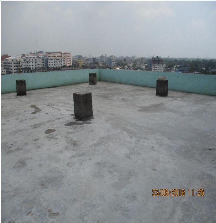
No water proofing membrane on roof top
