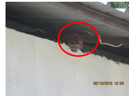
Weak support of truss
