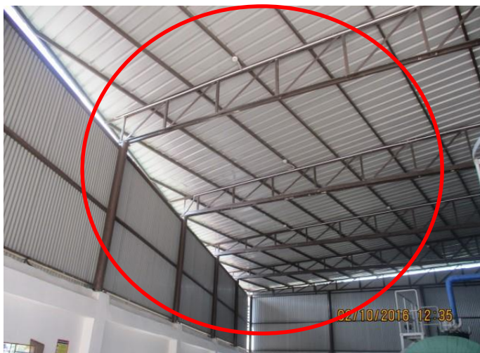
No bracing observed
