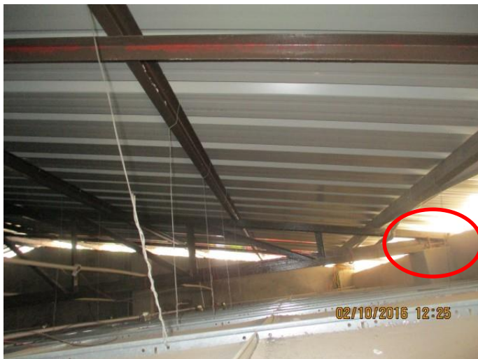
Weak connection between column & truss
