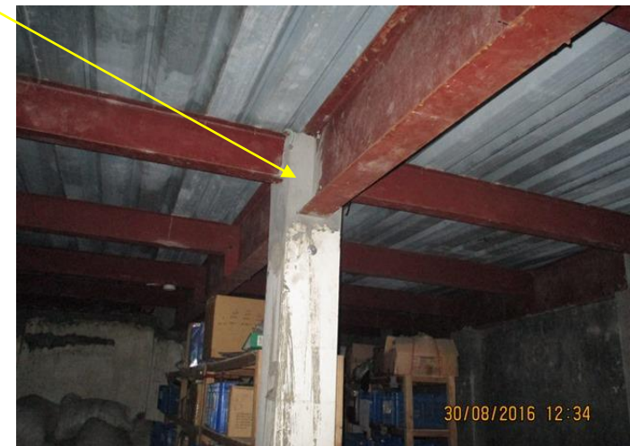
Connection with column is not clear. No details drawings was found for connection.
