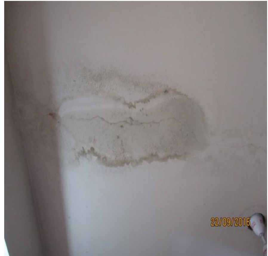
Water ingress through the crack of slab beside the north side stair case on 4 th floor.
