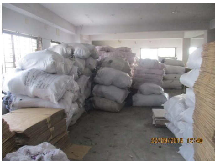
Over loaded area on 2 nd floor
