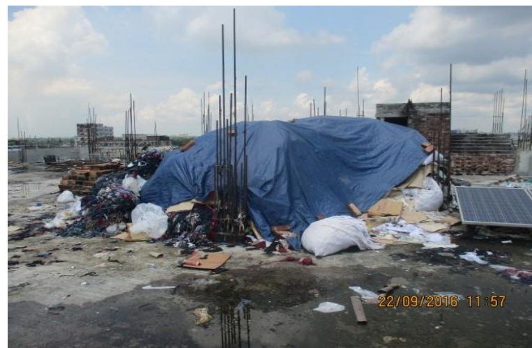
Over loaded area on roof top
