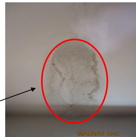
Cracks under the slab beside north side stair case
