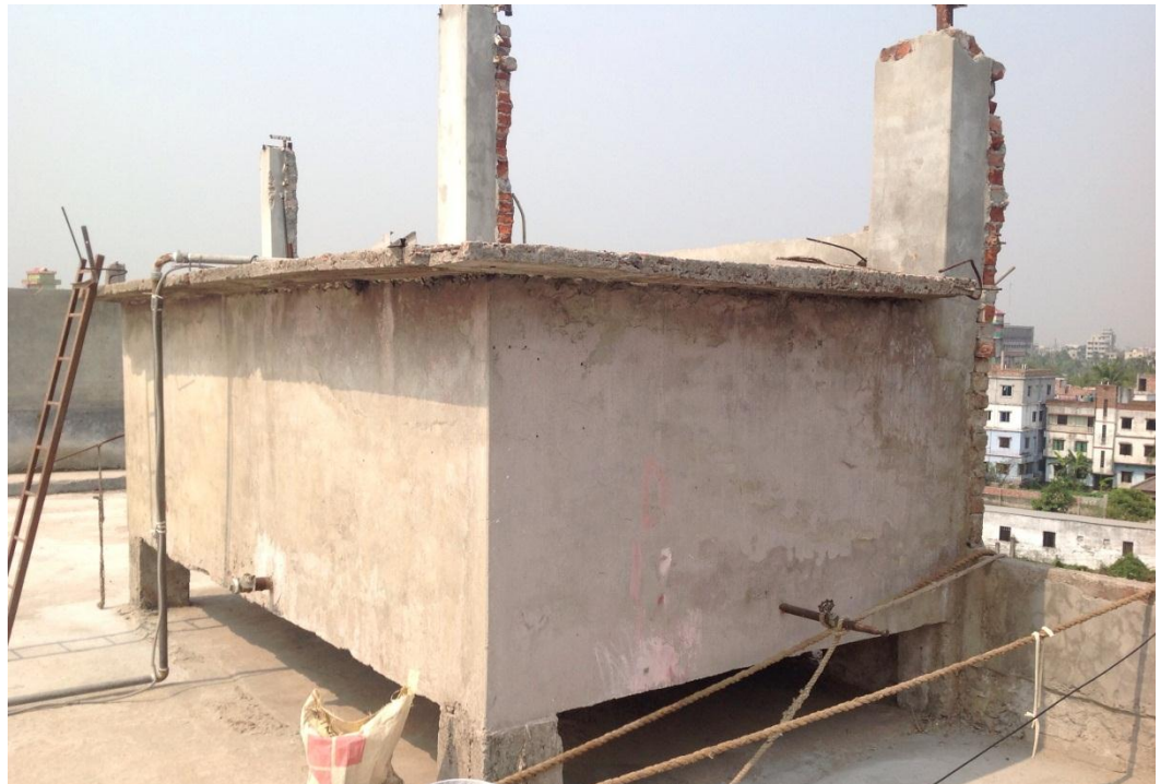
1.6m high water tank at roof level
