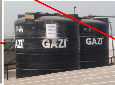
Plastic Water Tanks
