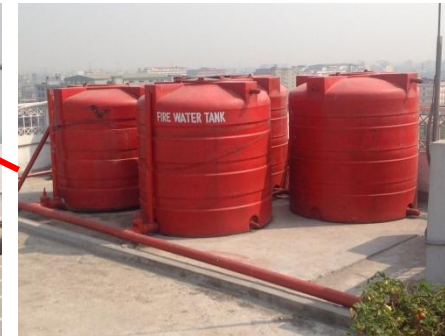
Plastic Water Tanks
