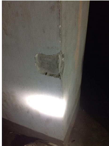
Tested Basement Column – Stone Chips
