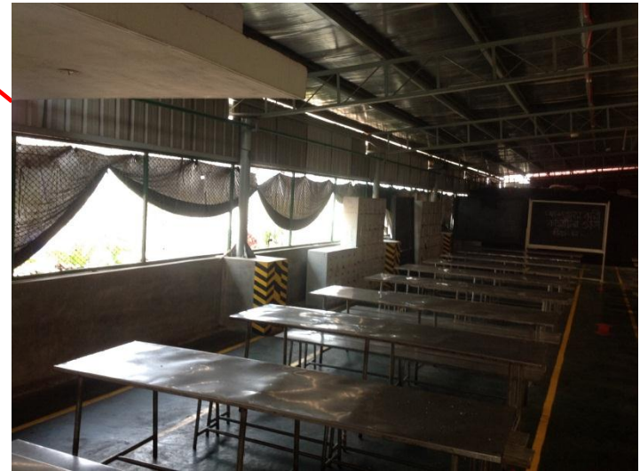
Steel structure on 6th Floor with no vertical bracing
