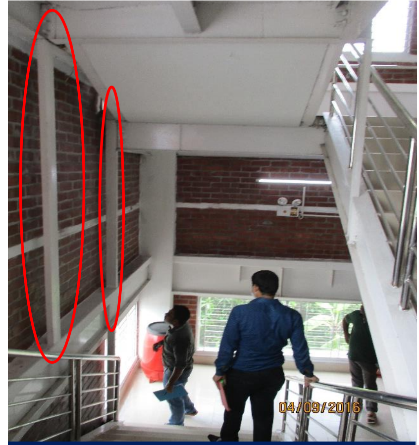
Extra steel column support steel stair
