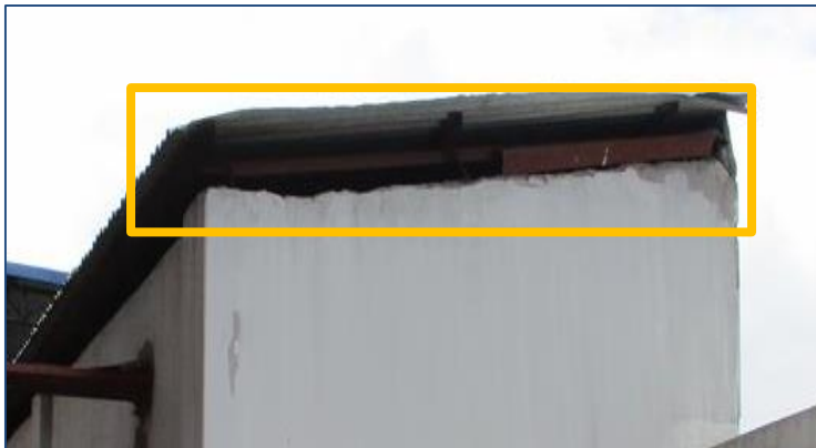
Poor connection between brick wall and steel roof.
