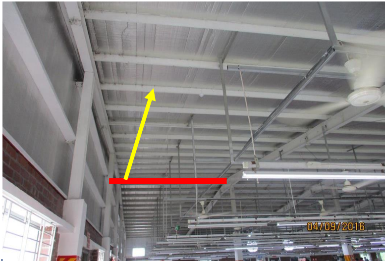
Missing compression strut at end bays
