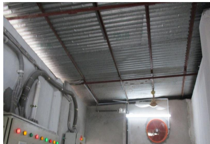
Non engineered steel roof of utility shed required to be checked against wind load.
