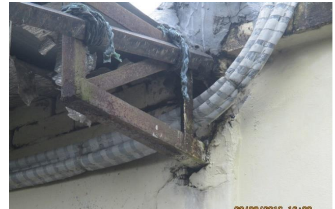
Corrosion in steel member
