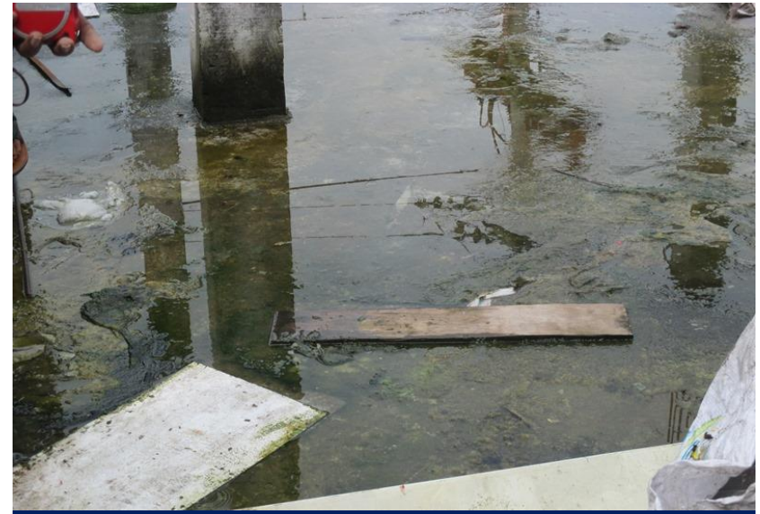
Water ponding on roof
