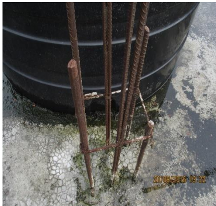
Unprotected column rebar
