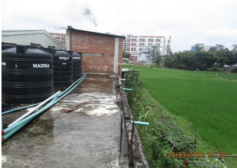
No edge protection on roof.
