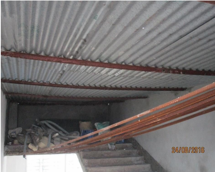
Deflection of steel member in roof of stair case.
