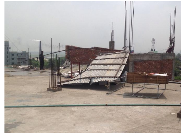
Apparently loose metal sheeting at Roof level
