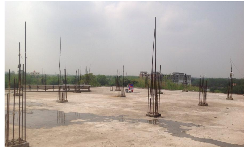
Lack of Fall Barrier to Roof
