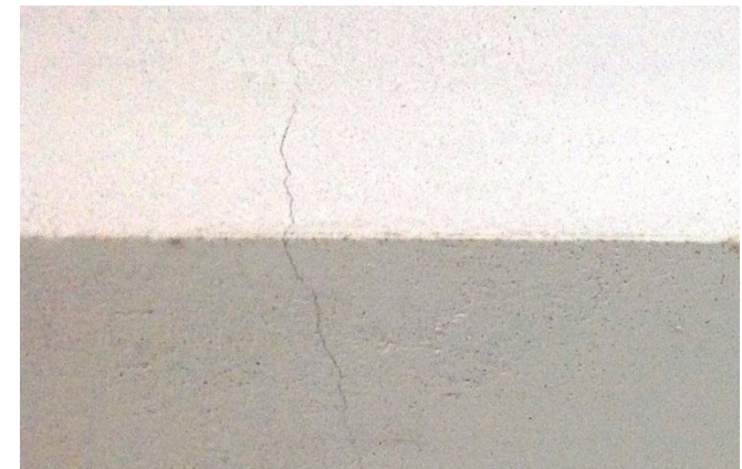
Cracking to underside of beam
