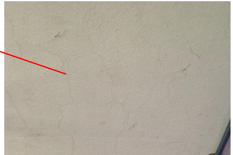
Roof slab soffit-observed cracks
