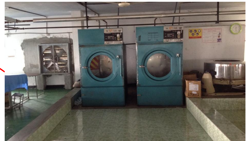
High loading (Dryers and plinth)
