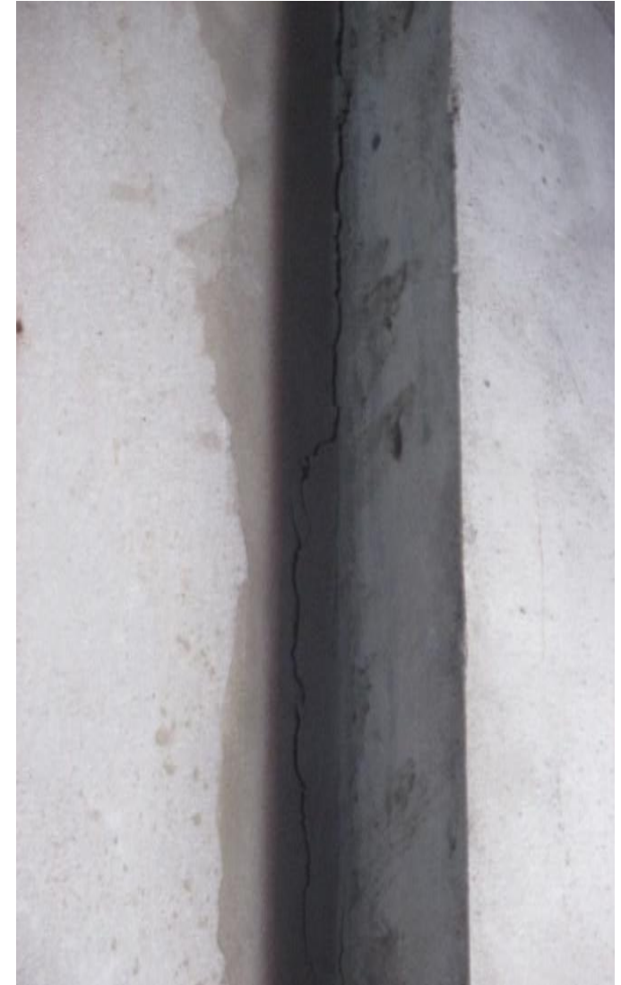
Loose bonding with column
