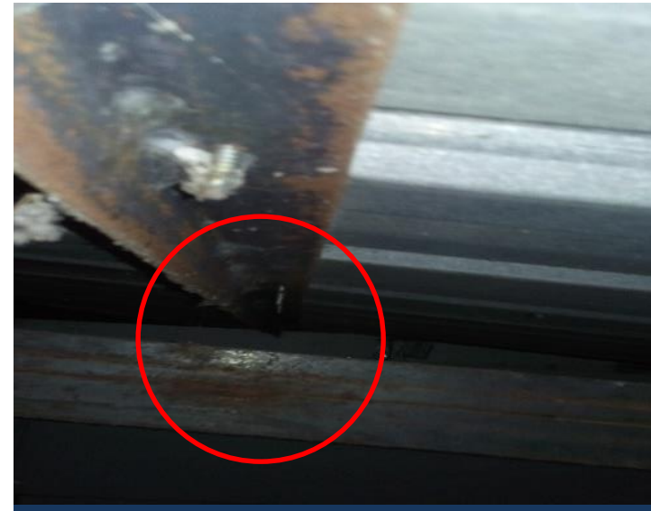
Purlins are not properly connected with steel rafter
