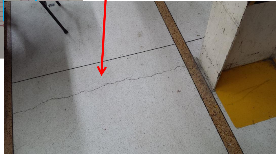
Cracking concrete slab
