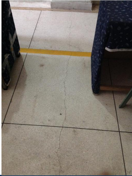
Cracking to ground floor slab
