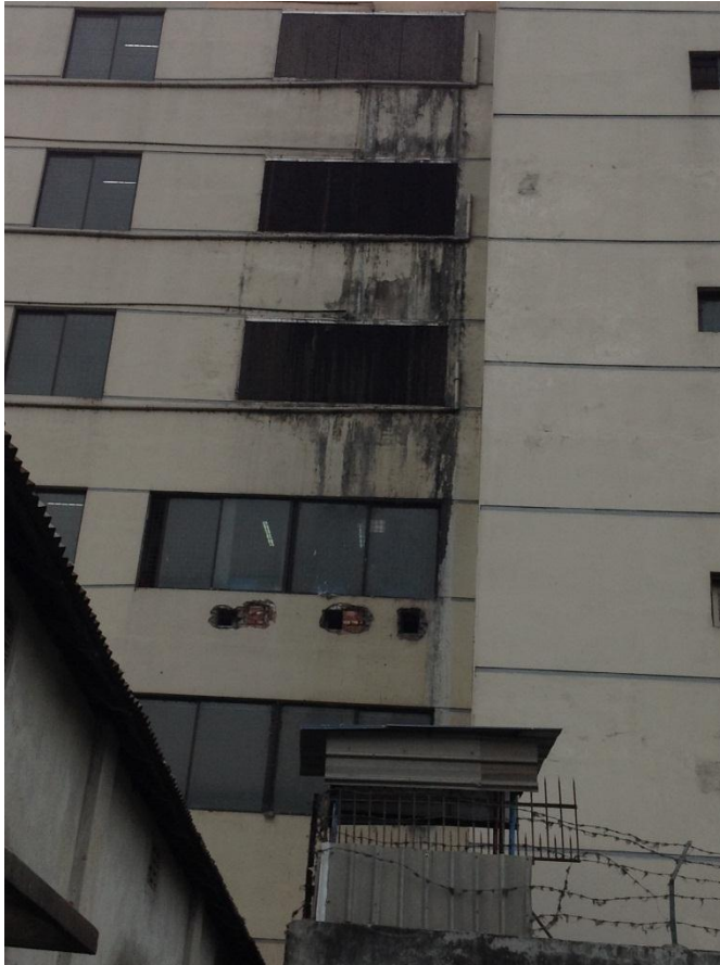
Water damage to façade on North Elevation
