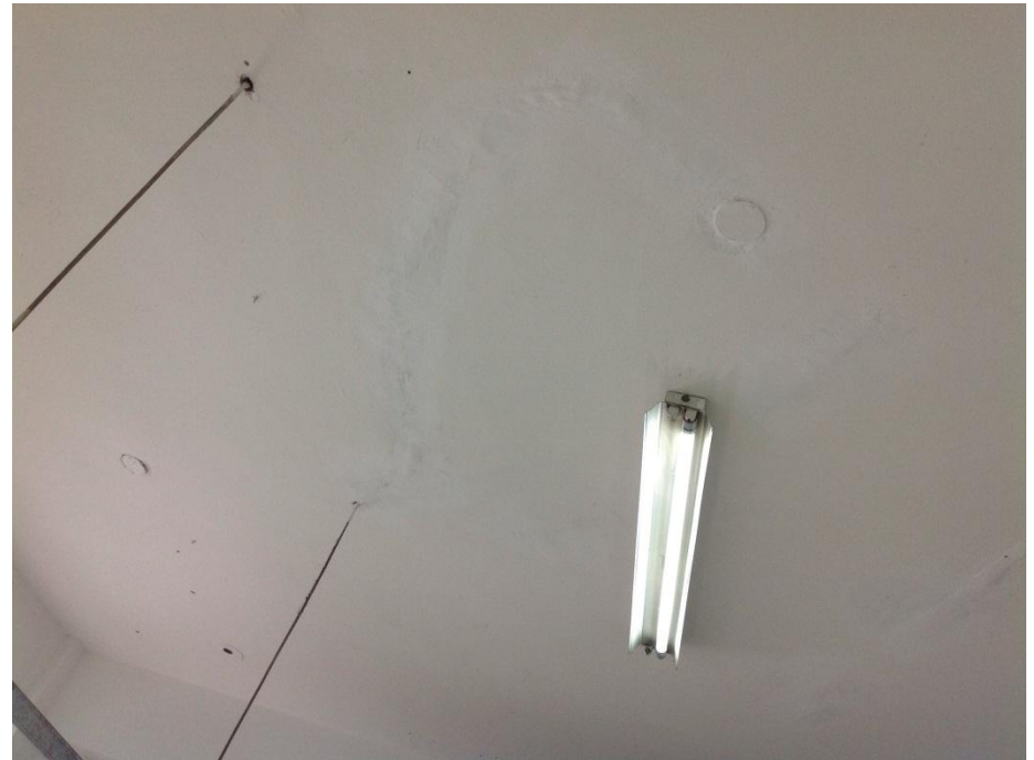
Water damage at soffit of roof slab
