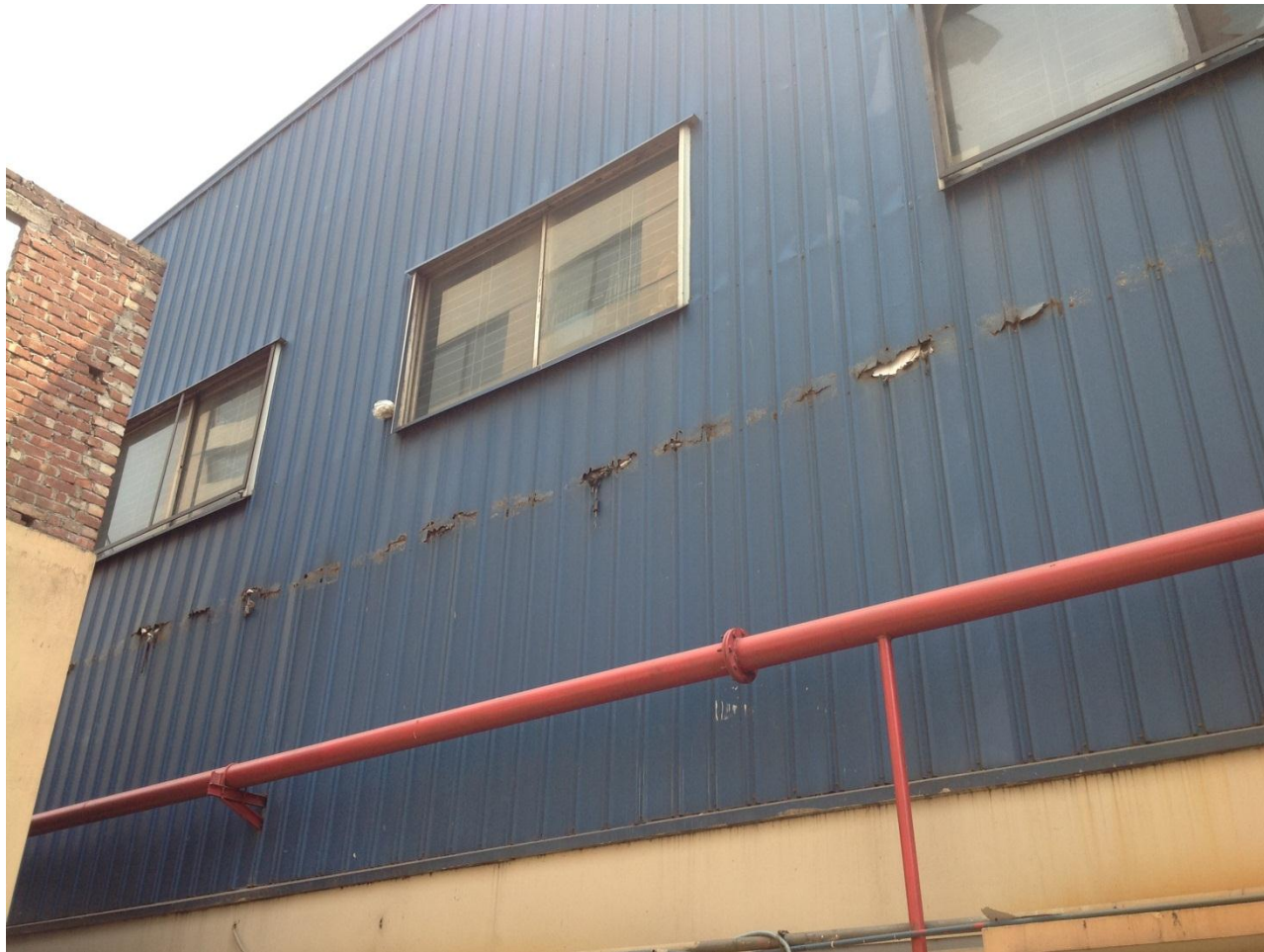
Damage to façade on the North Elevation
