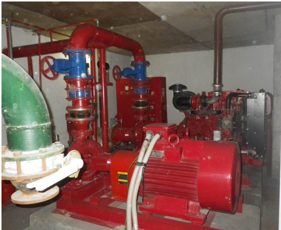
Photo 20 – Fire pump room with wood roof
