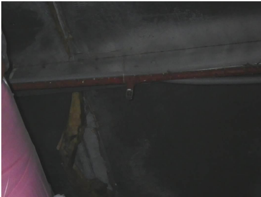
Photo 16 – Sprinkler system serving storage warehouse (Dyeing-1)
