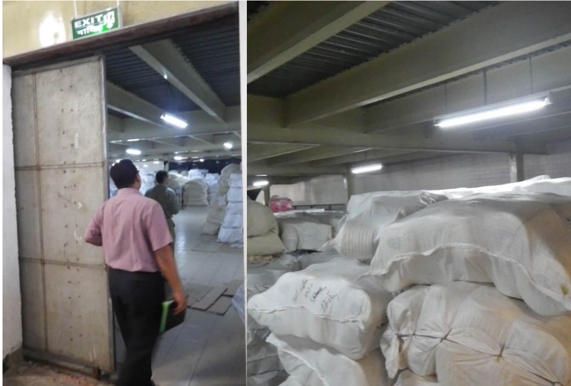
Photo 17 – Egress through storage warehouse, obstructed (Dyeing-2)
