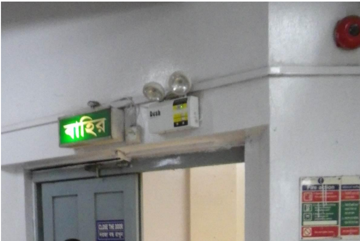
Photo 8 – Typical emergency lighting unit at exit stair (GMT-1)
