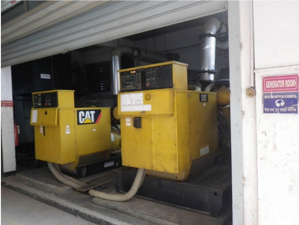
Photo 5 – Generator room (GMT-1)
