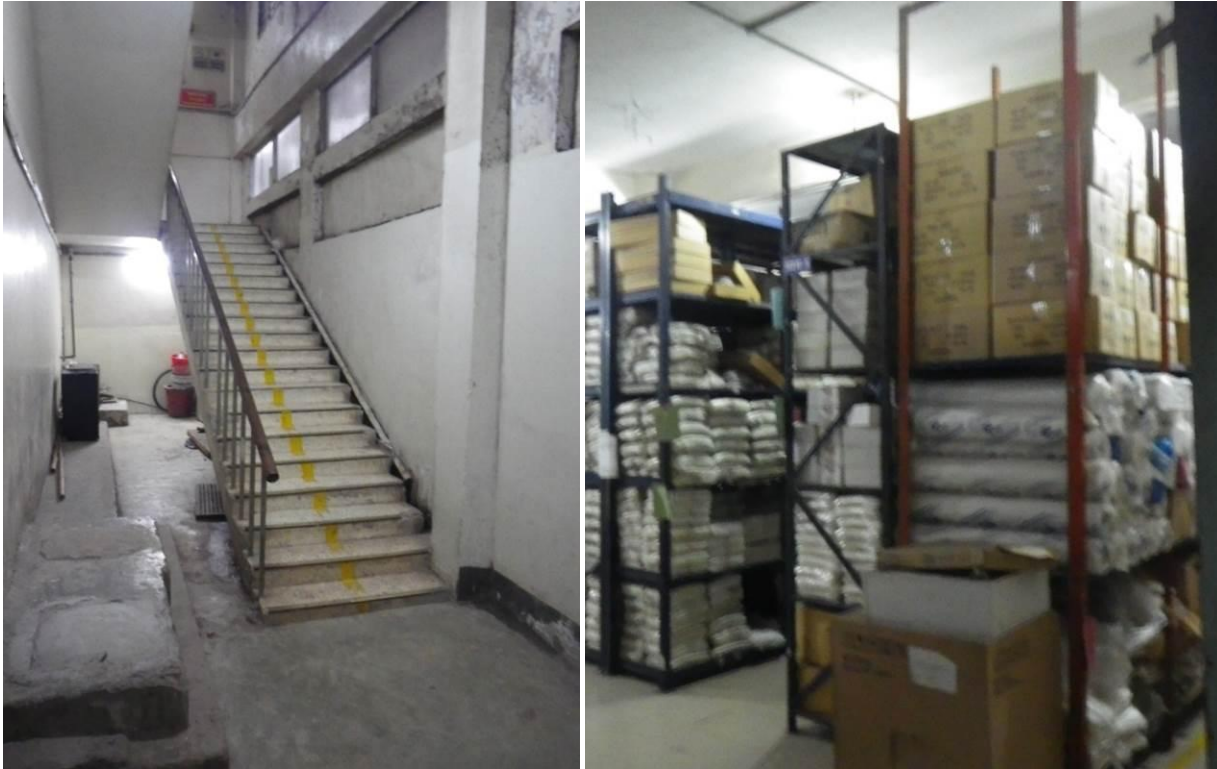
Photo 3 – Interior exit stair discharge open to storage areas (GMT-1)
