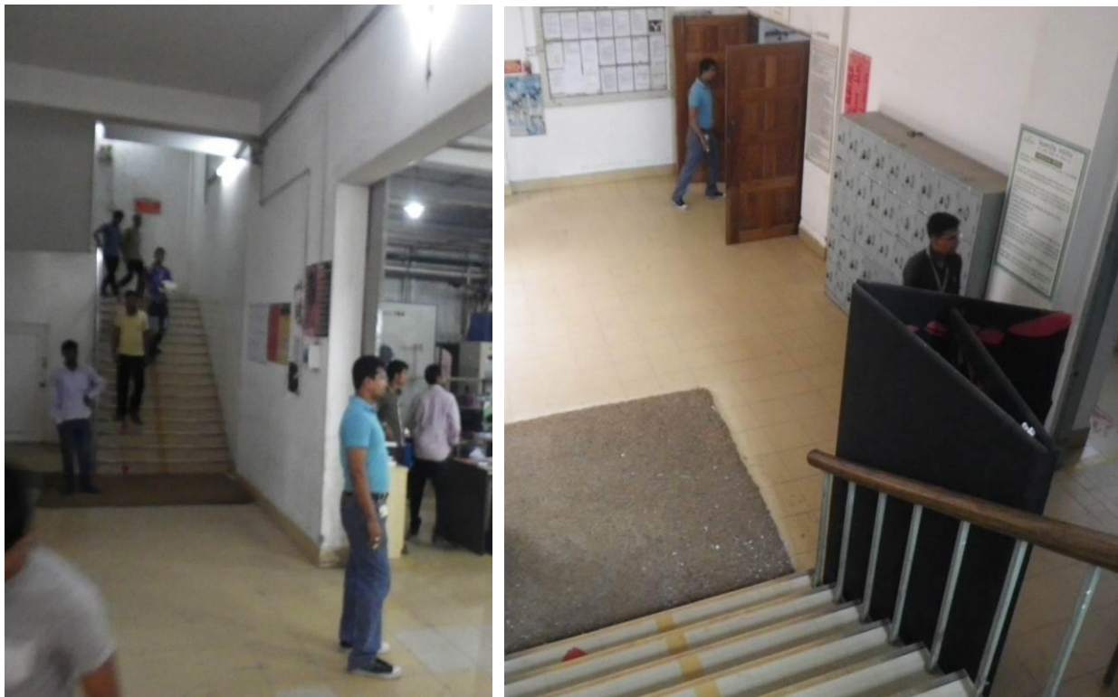
Photo 10 – Interior exit stair discharge open to storage and work areas (GMT-2)
