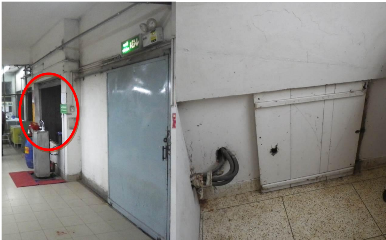
Photo 2 – Unprotected exit stair openings/penetrations (GMT-1, NW stair)
