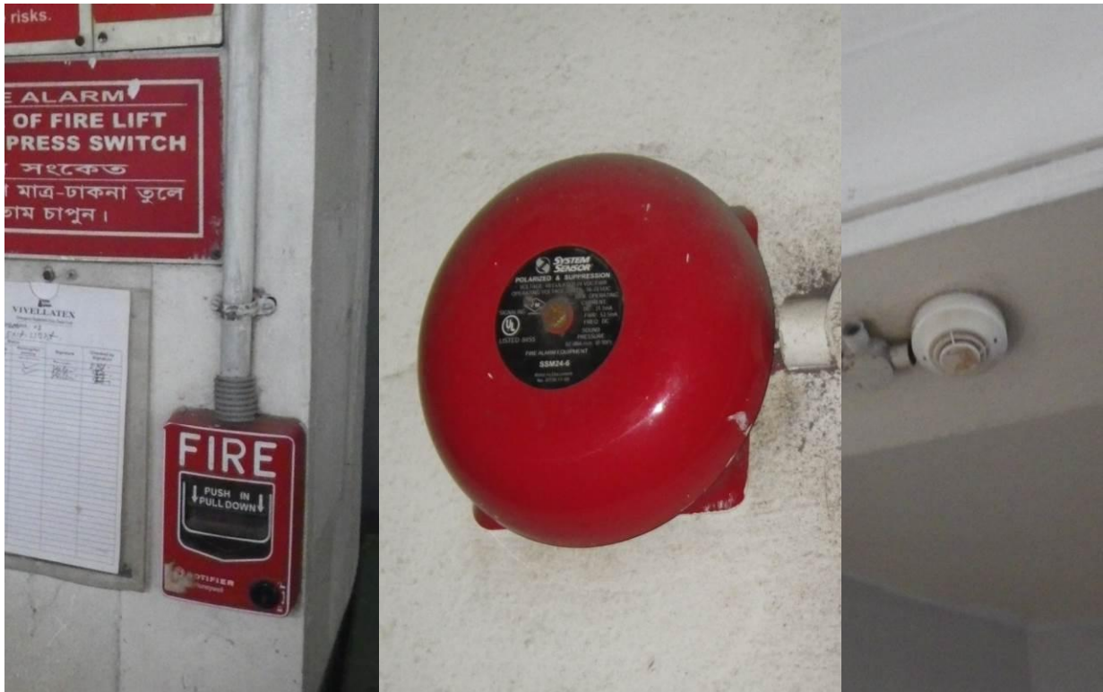
Photo 7 – Typical fire alarm devices (GMT-1)
