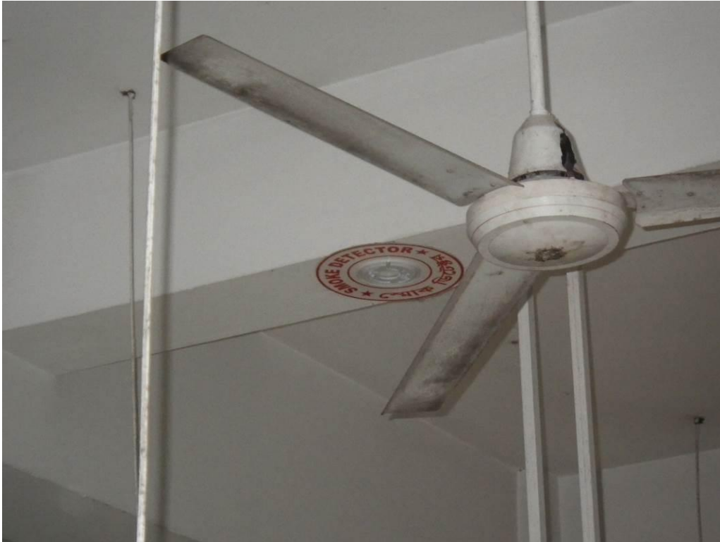
Photo 19 – Smoke alarm missing from base
