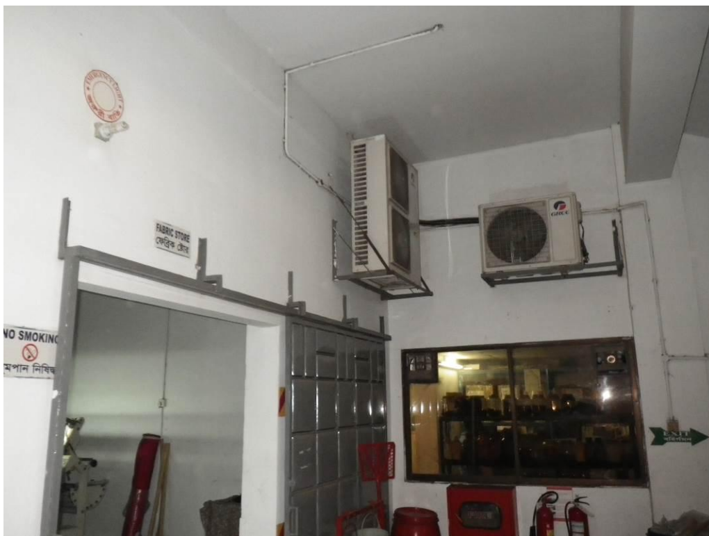
Photo 16 – Non-fire life safety equipment located in exit stair (HVAC fans)
