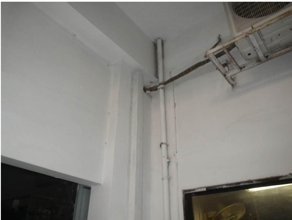
Photo 6 – Unsealed opening in ground floor of north exit stair
