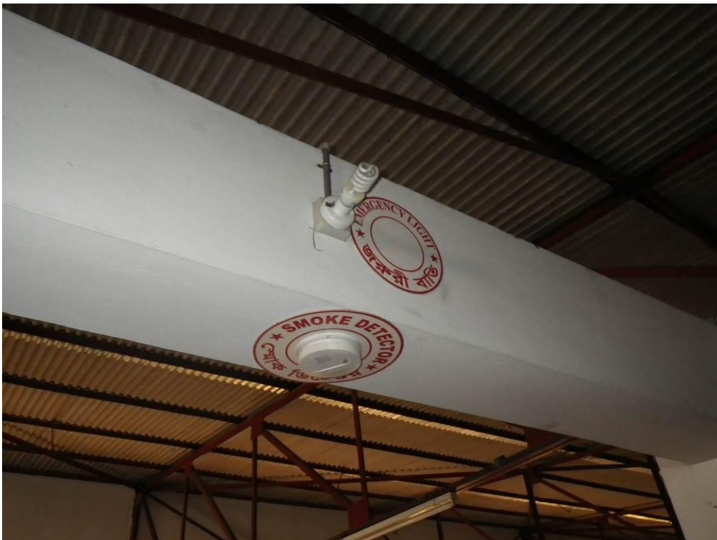
Photo 20 – Smoke alarm located well below the ceiling
