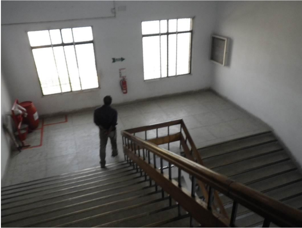
Photo 17 – Handrails provided on inside of exit stair only (typical)
