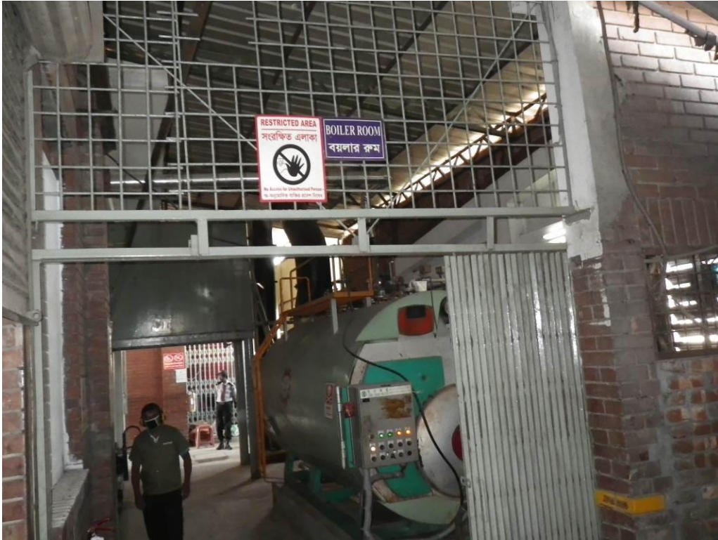
Photo 5 – Boiler room open to exterior egress path
