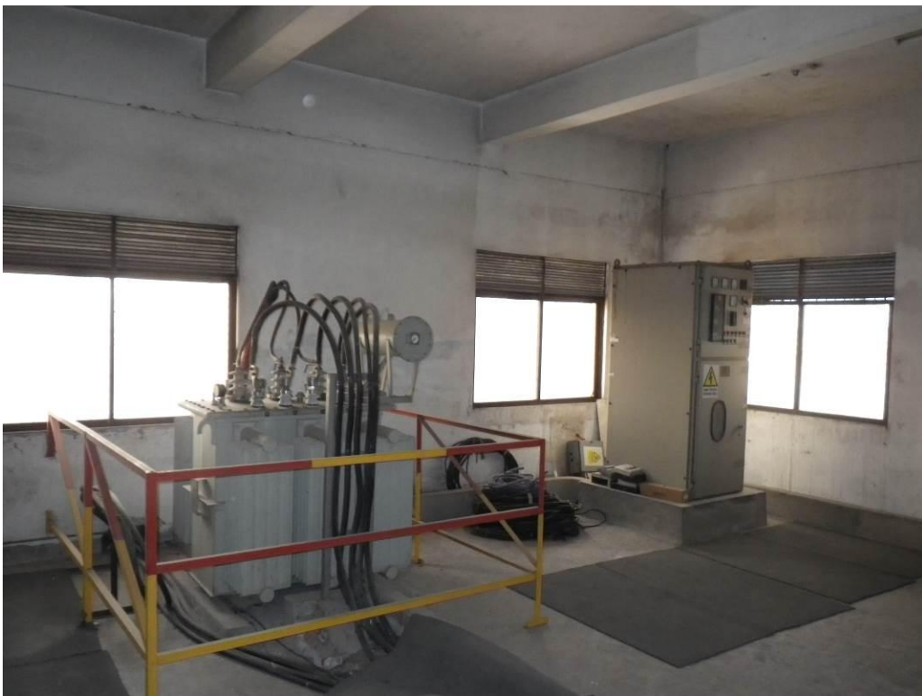
Photo 10 – Oil transformer and switchgear, nor fire separation
