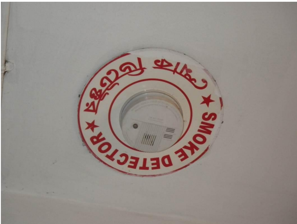
Photo 18 – Single-station smoke alarm (typical)
