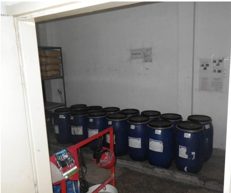
Photo 12 – Chemical storage room, no separation
