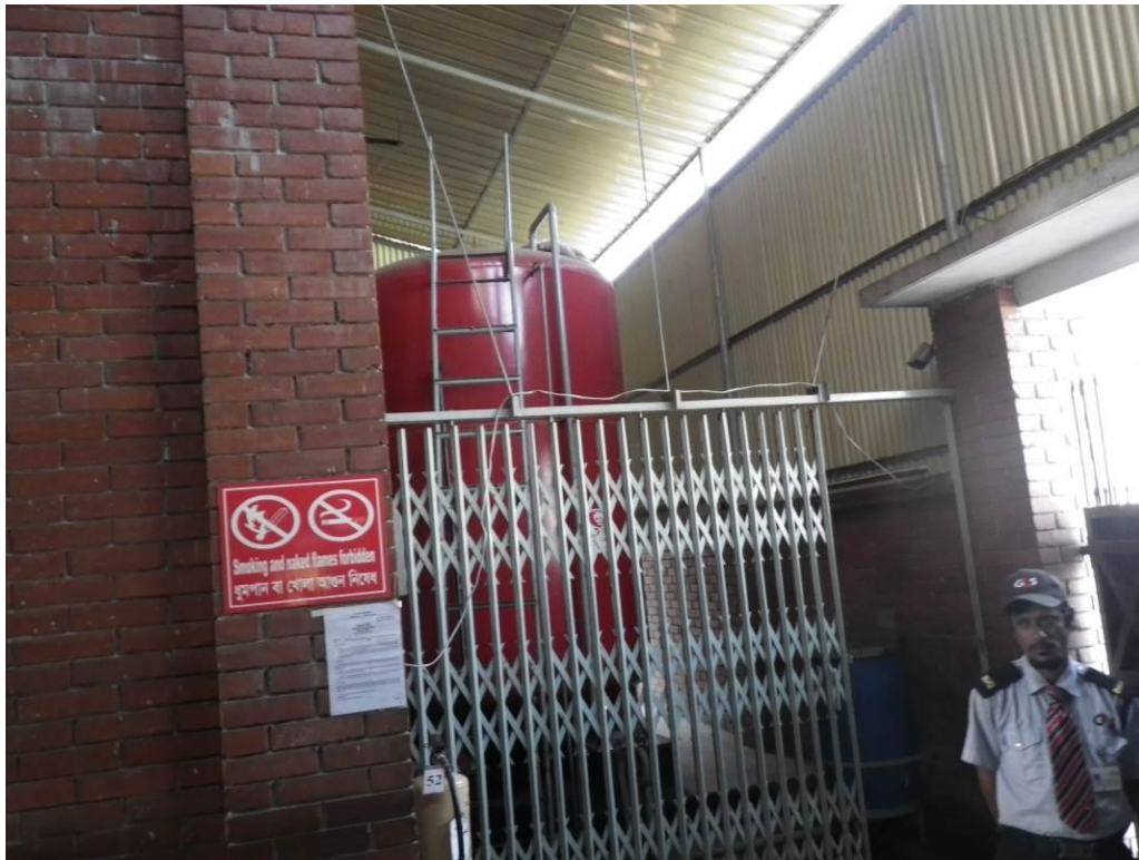
Photo 13 – Diesel fuel storage tanks, no separation
