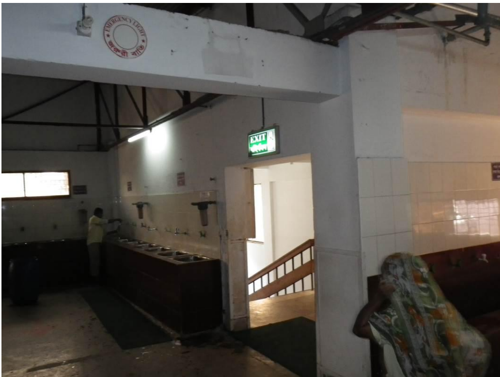
Photo 2 – Exit stair open to production area (typical)
