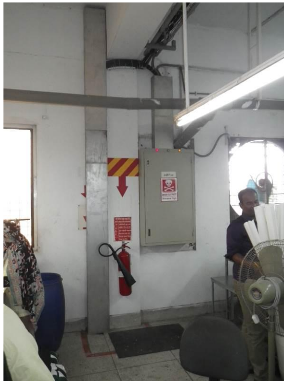
Photo 8 – Unsealed ceiling/floor penetrations, electrical riser
