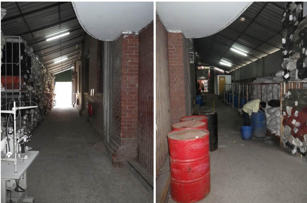
Photo 4 – Flammable and combustible storage in covered exterior egress path
