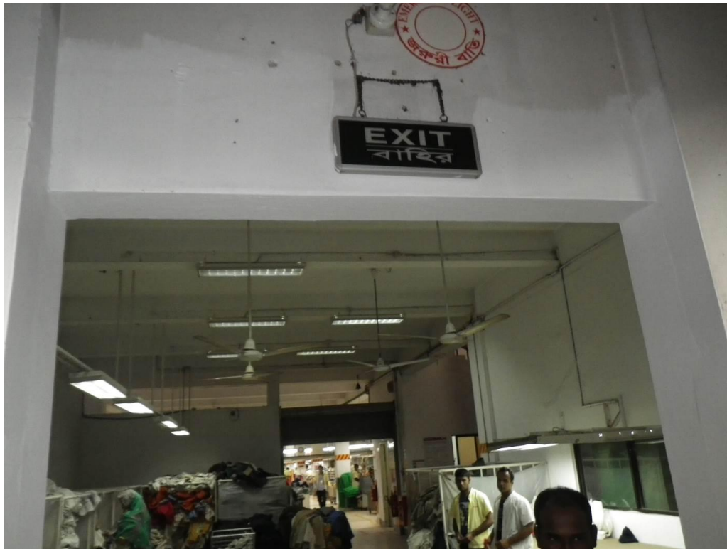
Photo 21 – Exit sign not illuminated
