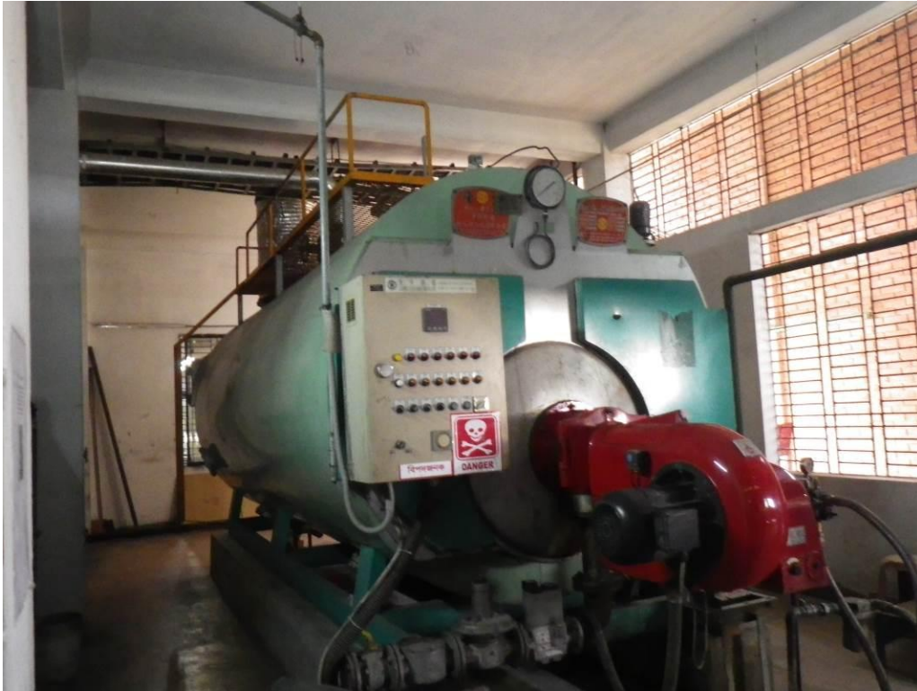
Photo 9 – Boiler room, no fire separation
