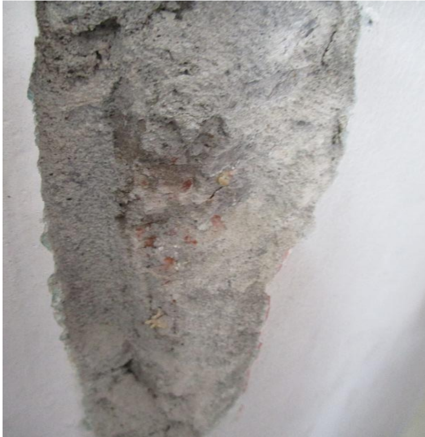
Brick chip aggregate observed
