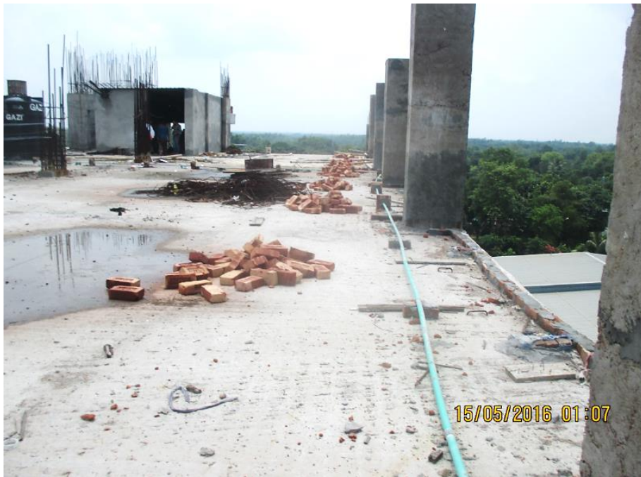
Missing edge protection on roof
