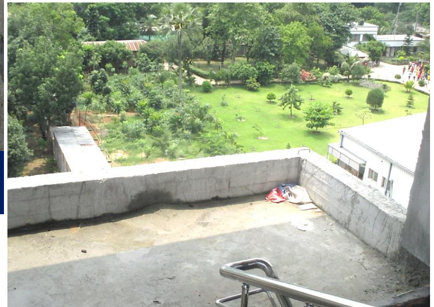
Missing edge protection on west side stair case
