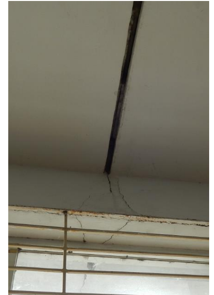
Cracking at expansion joint
