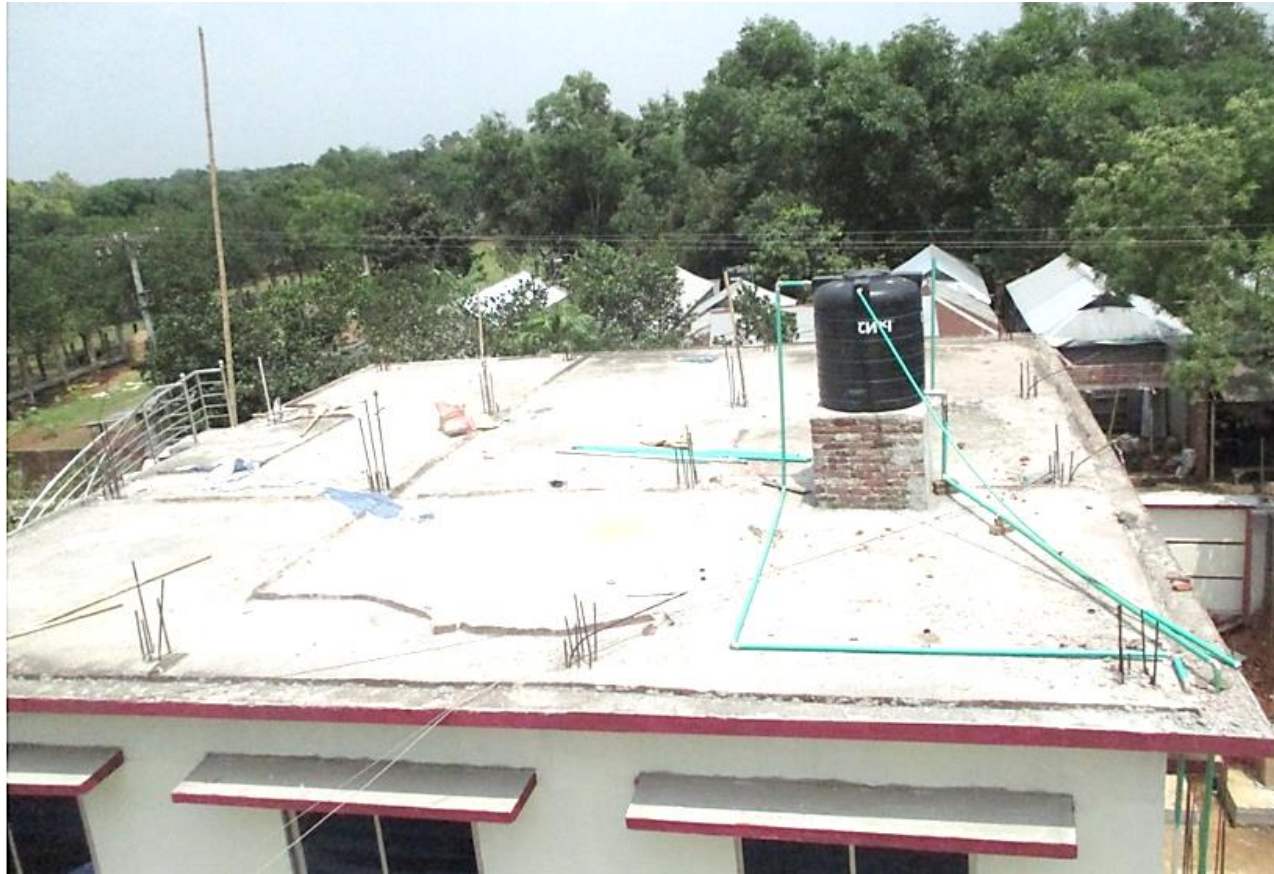
Missing edge protection on roof
