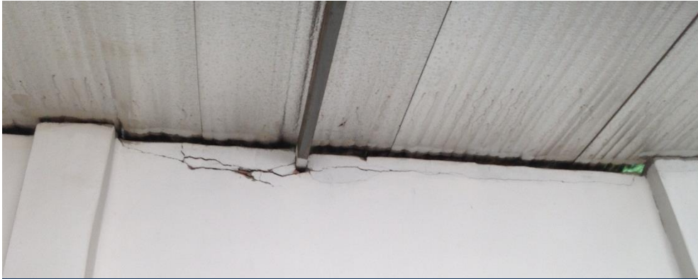
Cracking in masonry wall supporting roof beam
