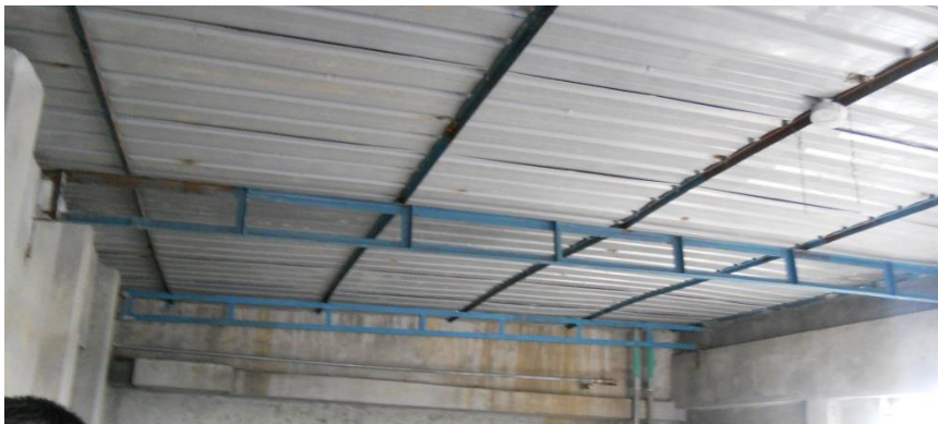
Lack of truss diagonals
