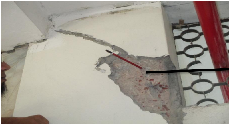
Column with eccentric beam found cracked Unclear Beam-Column arrangement.
