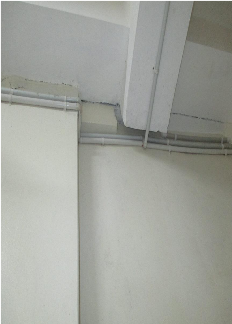
Beam offset to the column at 4 th Floor
