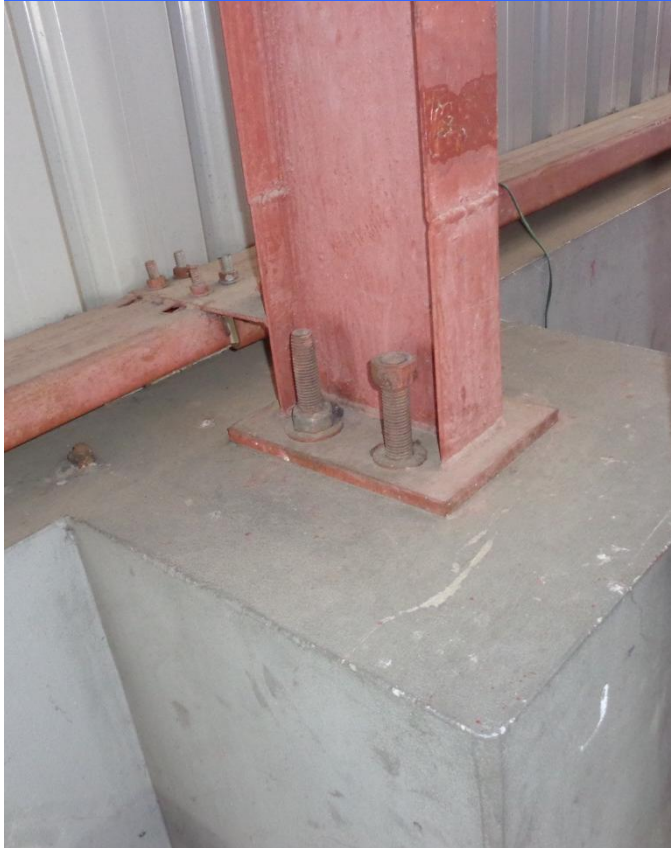
Nuts left loose on anchor bolts
