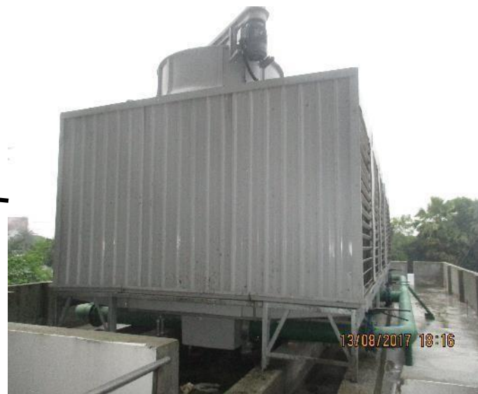
5000 Kg and 3500 Kg Cooling tower on roof top
