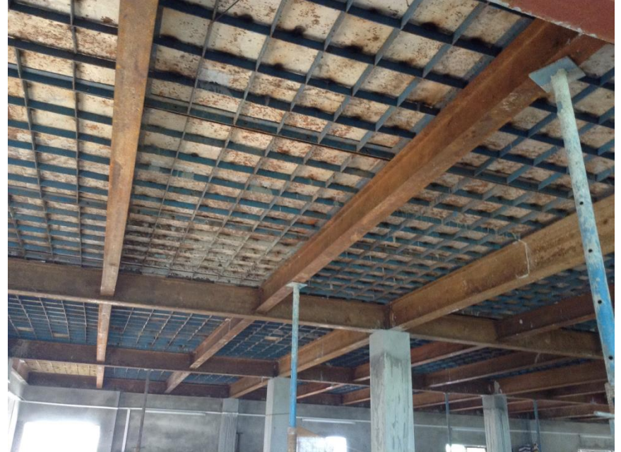
No vertical bracing observed
