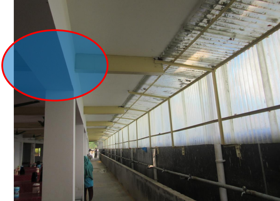
Discontinuous top reinforcement in the beam of ground floor
