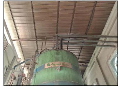
Jute Boiler Room
