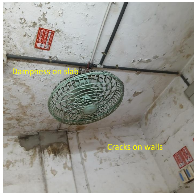
Fire Control Room
