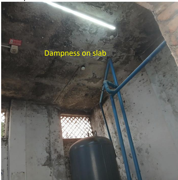
CMB Boiler Room
