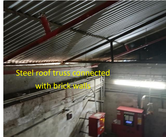
Fire Hydrant Room
