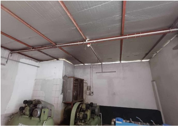
Shed-03: Compressor Room
