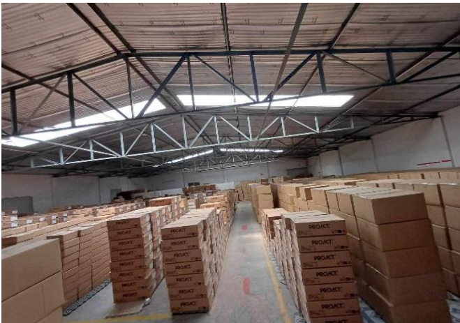
Inadequate framing in long direction
