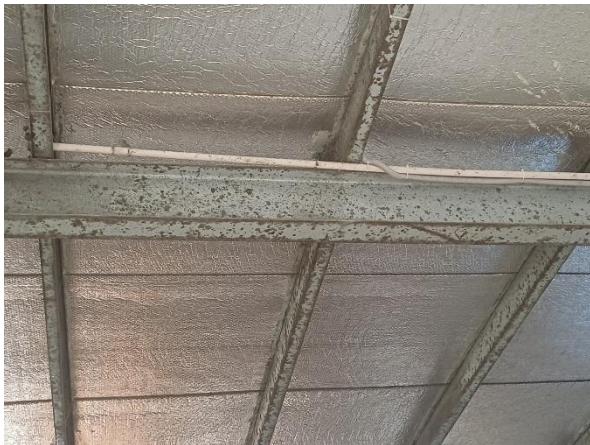
Corrosion on the rafter of the Dining Shed
