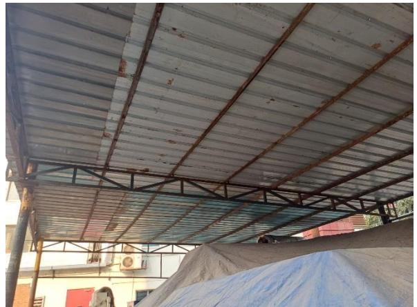
Corrosion on the truss & purlin of the Temporary Generator shed
