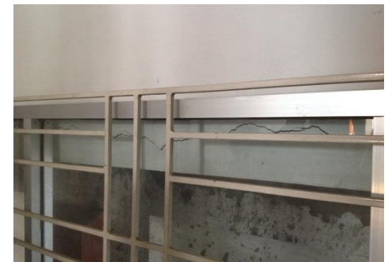
Cracking in staircore
