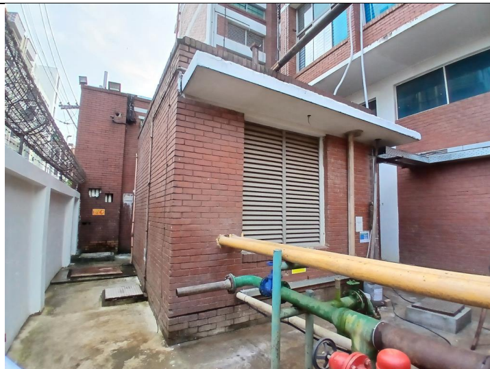
Building-5: RMS Room
