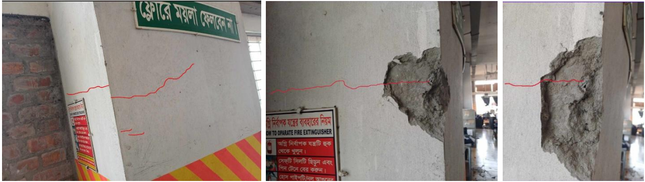
Hairline crack on the column
