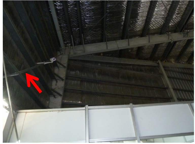
Loose wall cross bracing
