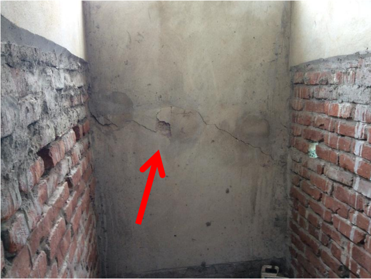
Examples of cracking to brick walls
