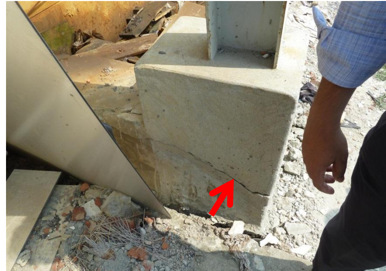
Failure of shallow footing to stairs
