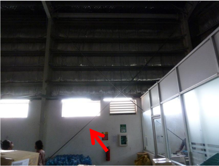
Loose wall cross bracing
