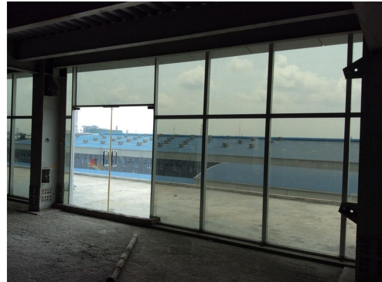
Example of cross bracing omitted on account of door
