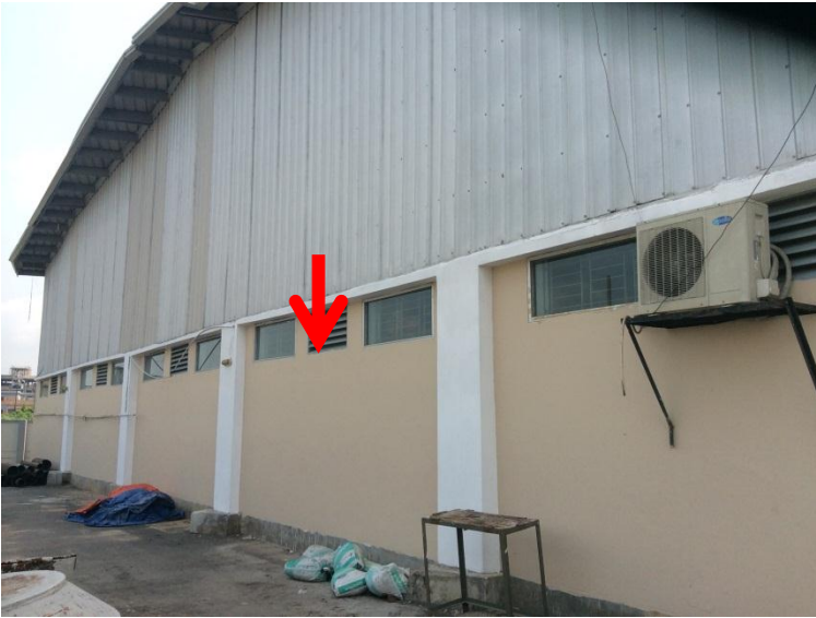
As constructed, lateral support to tops of brick walls is not clearly defined
