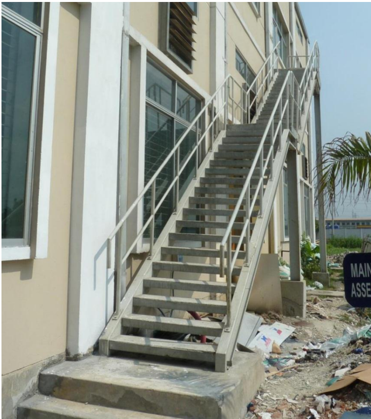
Settlement of ground beneath shallow footings to stairs
