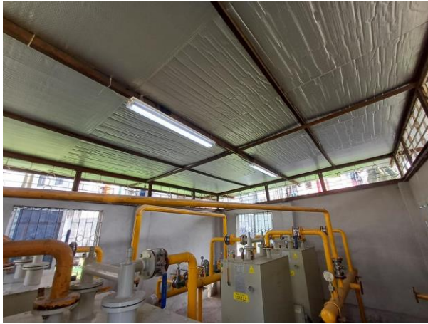
LPG Storage & Vaporizer Room
