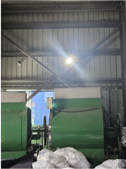
Misaligned vertical bracing
