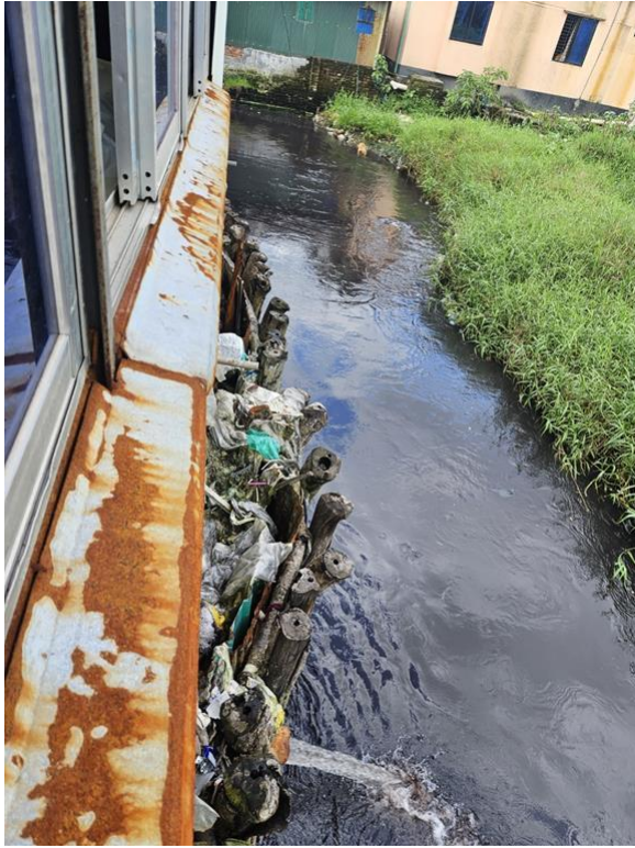
Tilting of wooden shore pile
