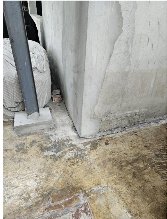
Settlement of the floor and cracks
