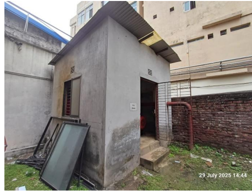
Shed-6: Fire Pump room
