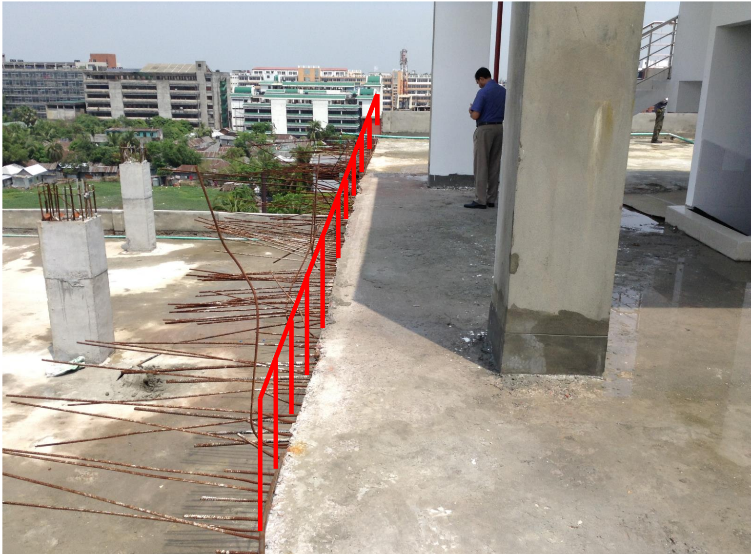
Lack of handrails on the 7 th floor.
