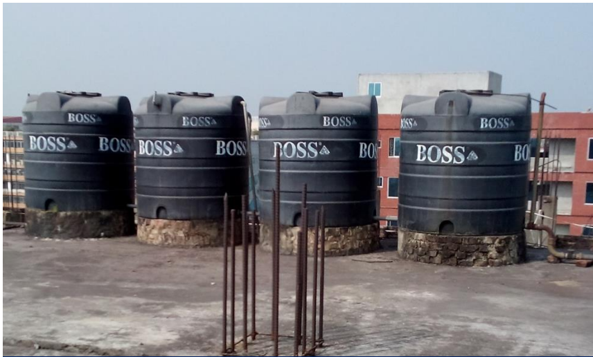
4, 2000 lt water tank on roof
