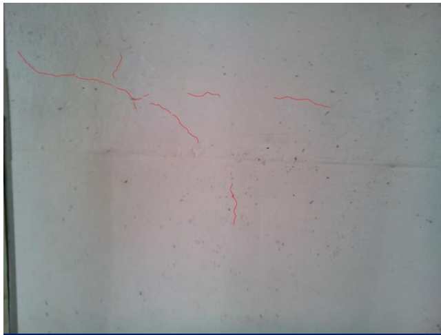
Cracks on 6 th floor roof slab
