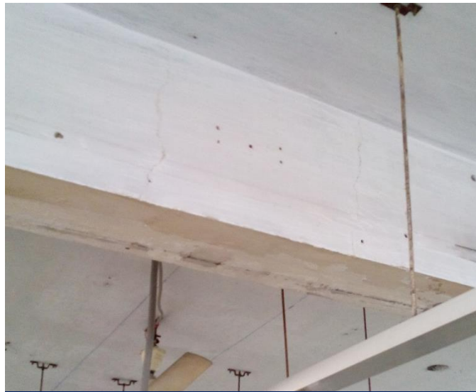
Cracks on Beams of 5 th floor roof slab
