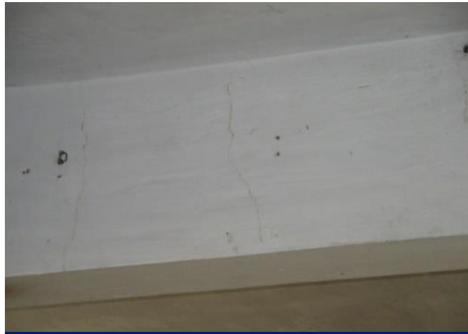
Cracks on Beams of 5 th floor roof slab
