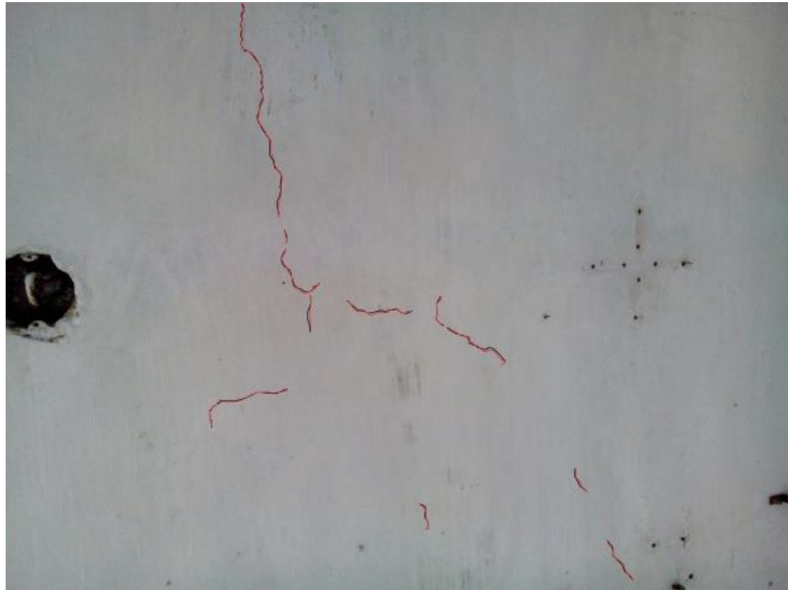
Cracks on 5 th floor roof slab
