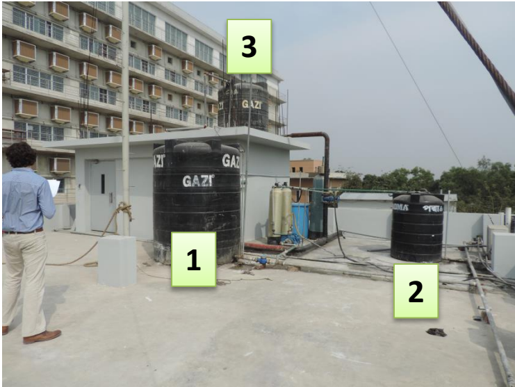
Water Tanks on the roof
