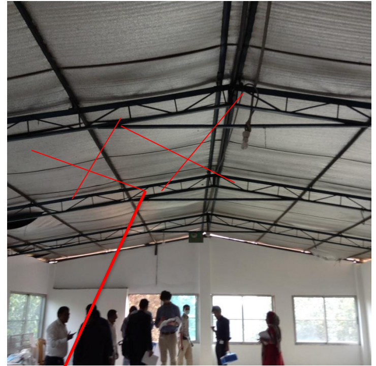
Lack of bracings on the metal roof
