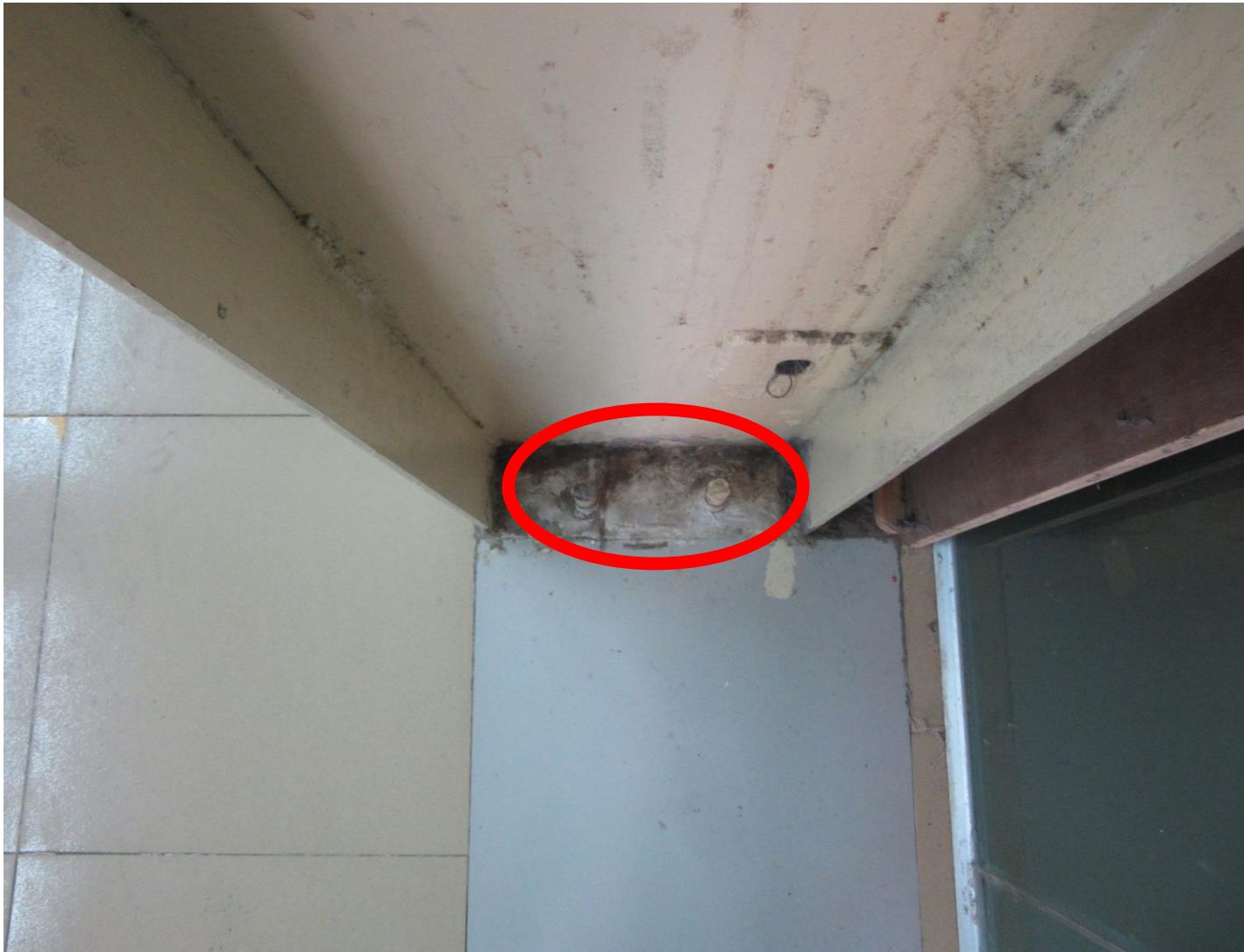
Nuts could not be seen at the base plate connection.
