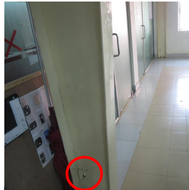
Missing Vertical Bracing
