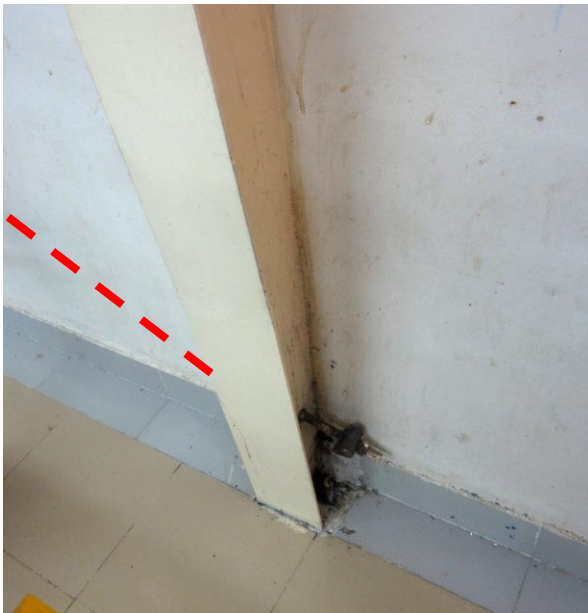
Missing Vertical Bracing
