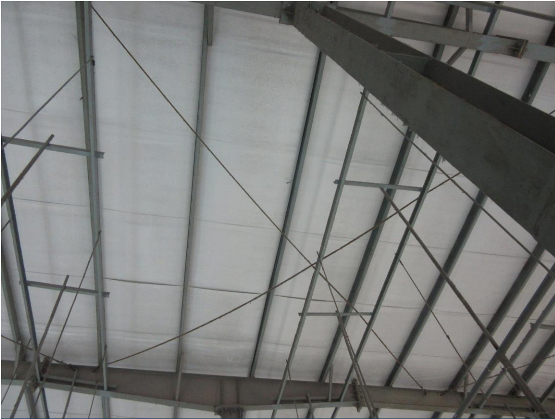
Sagged Horizontal Bracing Cables
