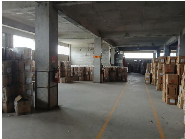
Trolley impact and surface damage on columns
