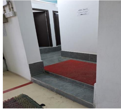
Buildup at the toilet zone
